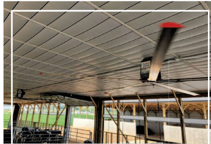
HVLS CEILING FANS
