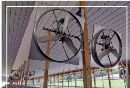
EXHAUST & CIRCULATING FANS
