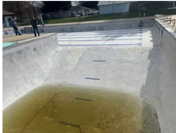
Patches of past plaster repairs near The deep end of the pool
