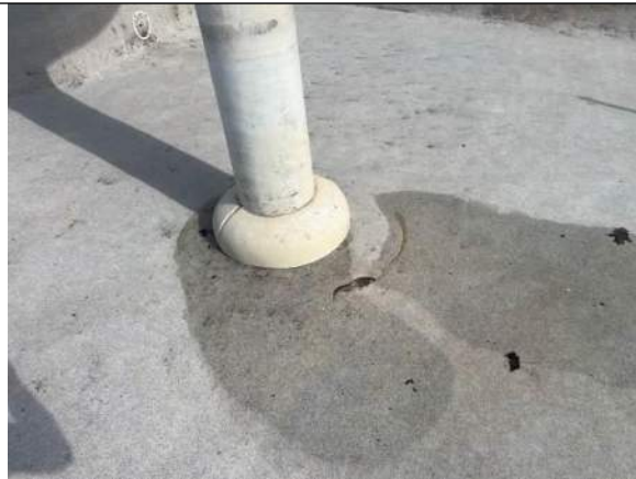
Water leak around the mushroom column.
