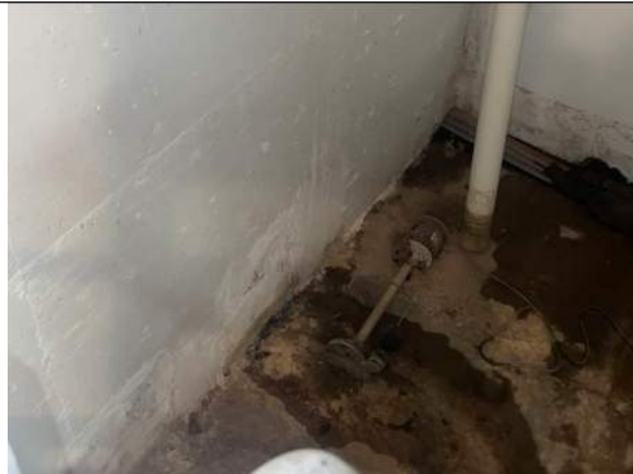
Water leak near west side of east pump house wall
