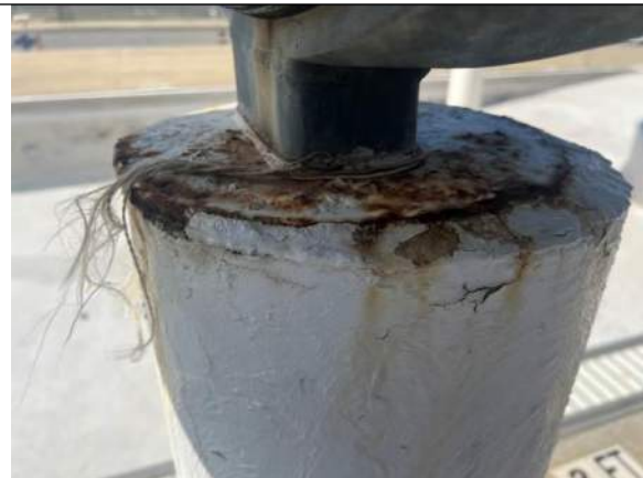
Rusted steel and anchor bolts at the waterslide supports.
