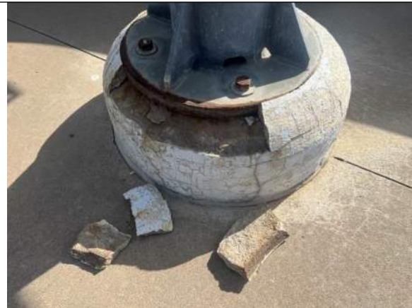
Cracks in concrete pilaster.
