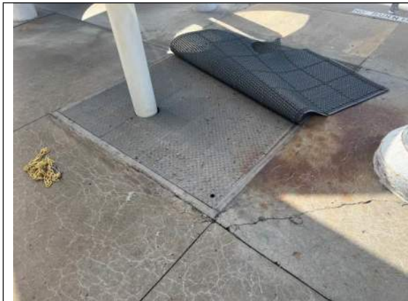
Shifting of the concrete pool deck
