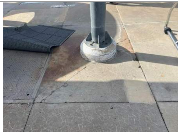
Shifting and cracks of the concrete pool deck
