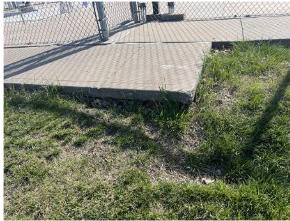
Voids below concrete sidewalk
