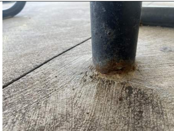
Signs of rust at bottom of steel column
