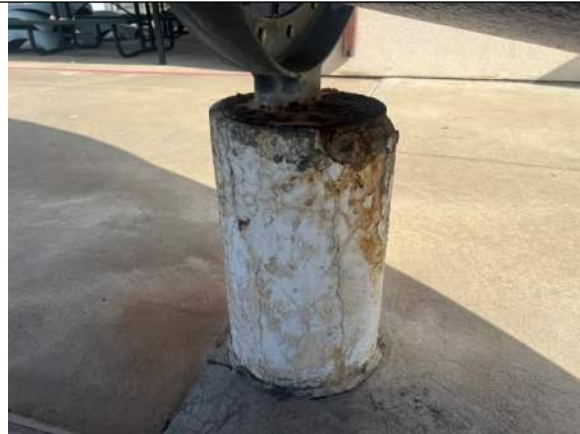
Rusted steel and anchor bolts at the waterslide supports. Cracks in concrete pilaster.
