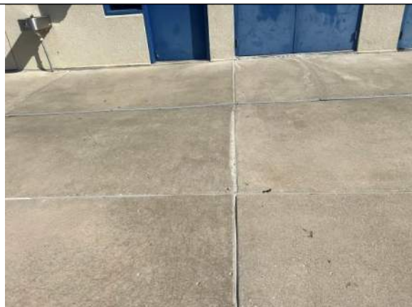
Shifting of the concrete pool deck
