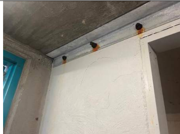
Rusted bolts at angle on the Wall inside the pump house
