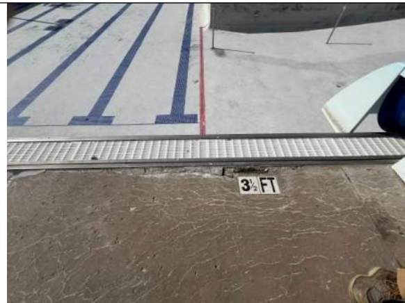
Concrete deterioration at the northeast corner of the pool deck
