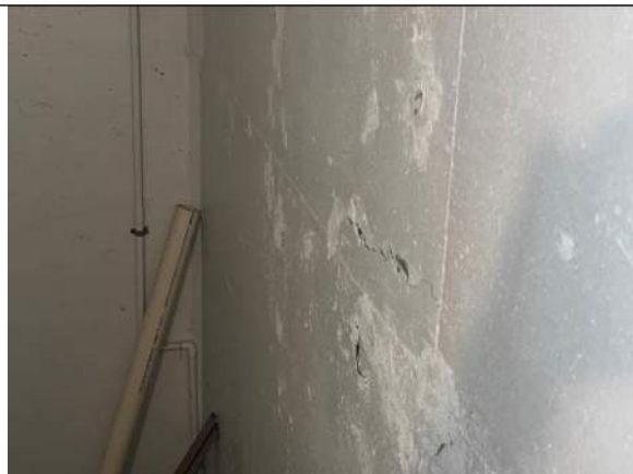
Horizontal cracks in pump house concrete wall
