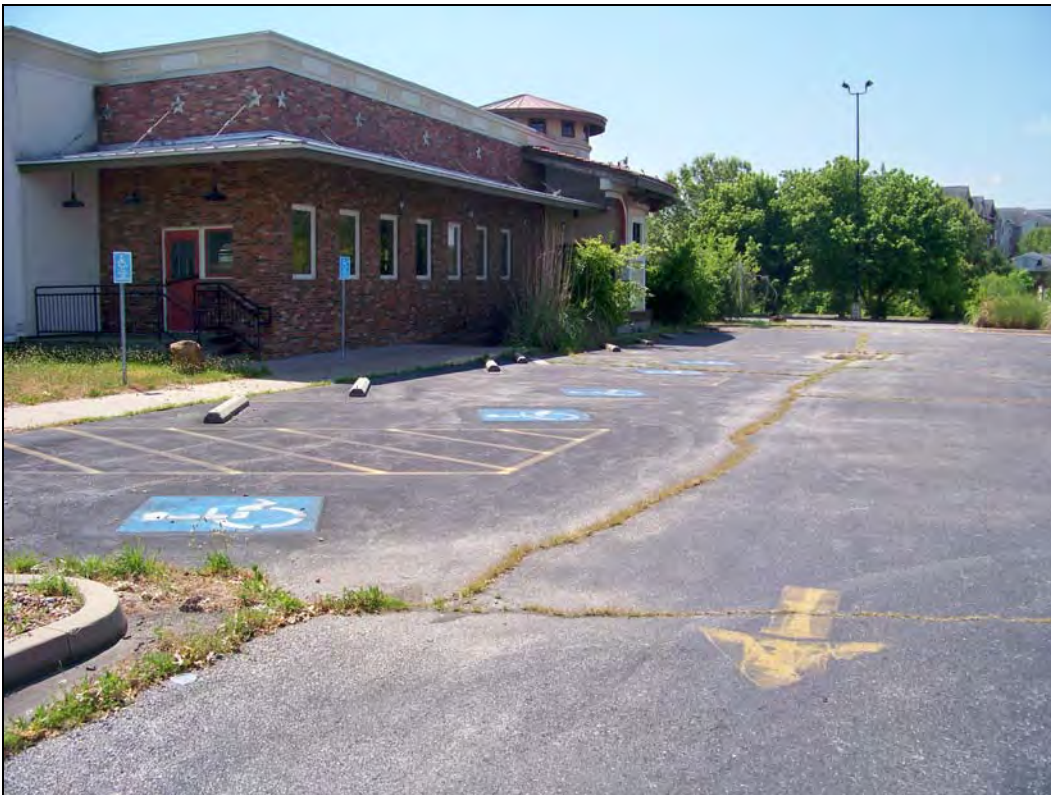
Parcel No. 04-4.0-19-000-000-005.007 – looking south – deterioration of pavement
