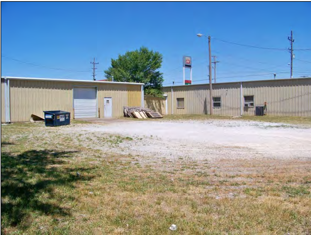
Parcel No. 04-4.0-19-000-000-006.000 – looking northwest – deterioration of improper parking surface; unenclosed trash area; trash/debris
