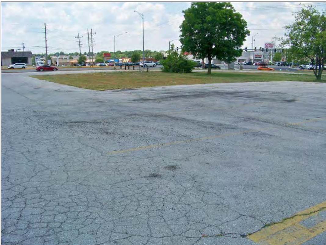
3209 S. Range Line Road – looking northwest – deterioration of pavement
