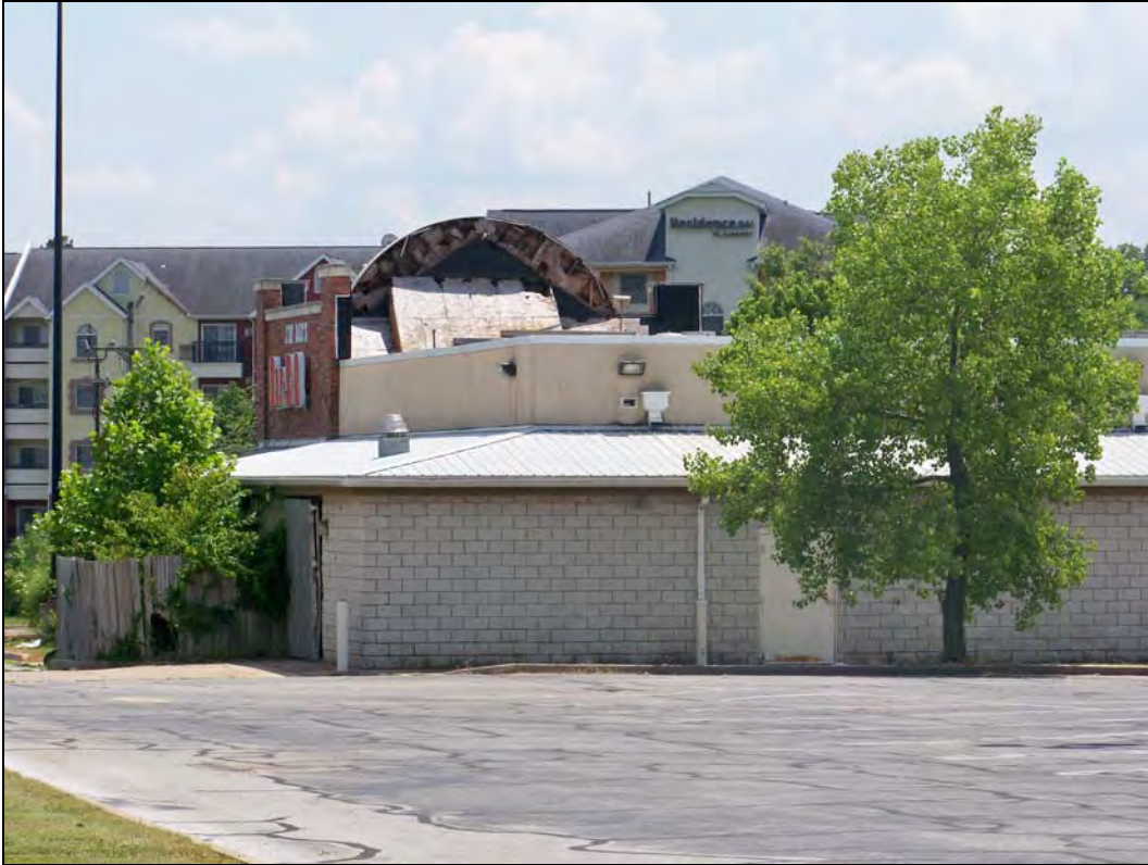
Parcel No. 04-4.0-19-000-000-005.007 – looking south – deterioration of roof
