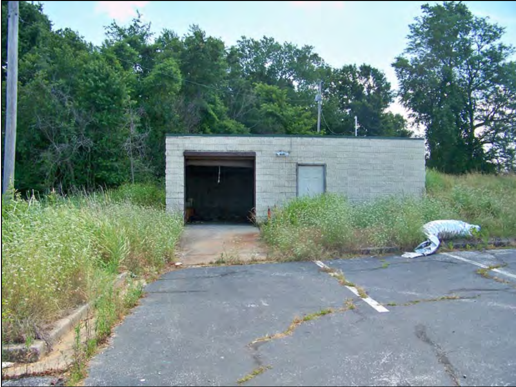
Parcel No. 04-4.0-19-000-000-005.003 – looking east – deterioration of ancillary building; overgrown vegetation; trash/debris
