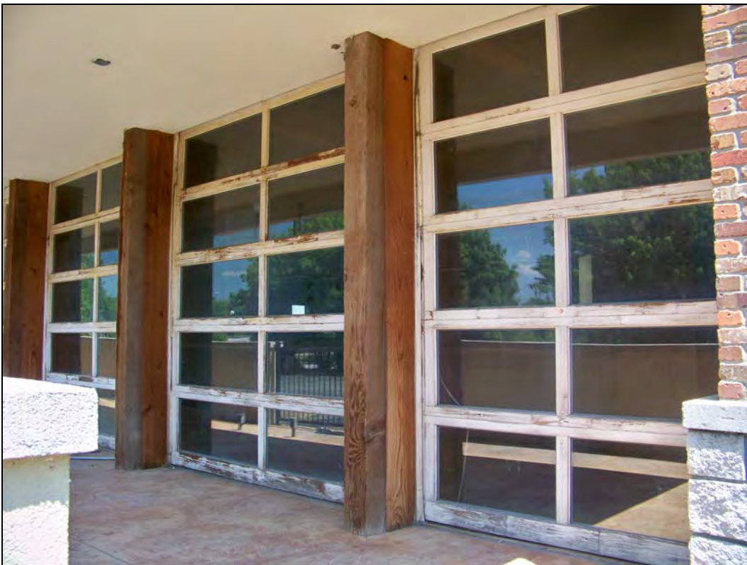
Parcel No. 04-4.0-19-000-000-005.007 – looking northwest – failure of finishes
