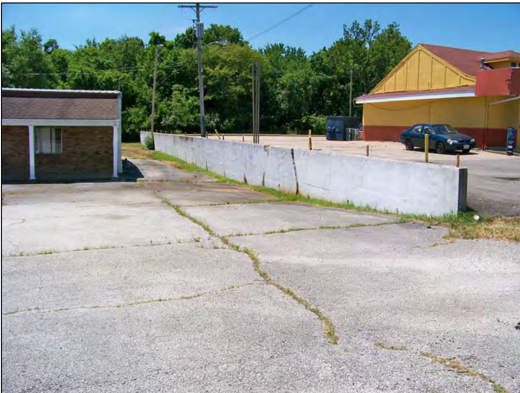
Parcel No. 04-4.0-19-000-000-006.000 – looking southwest – deterioration of pavement, wall
