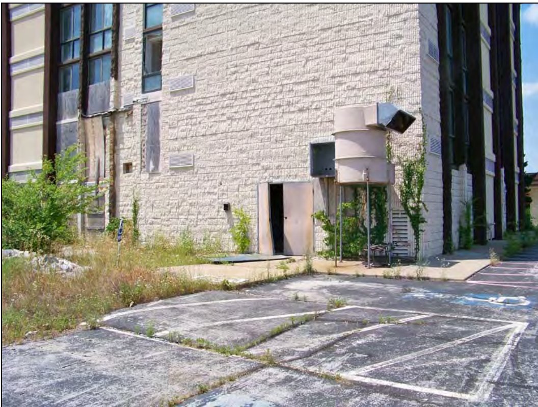
Parcel No. 04-4.0-19-000-000-005.003 – looking west – boarded windows; damaged doors
