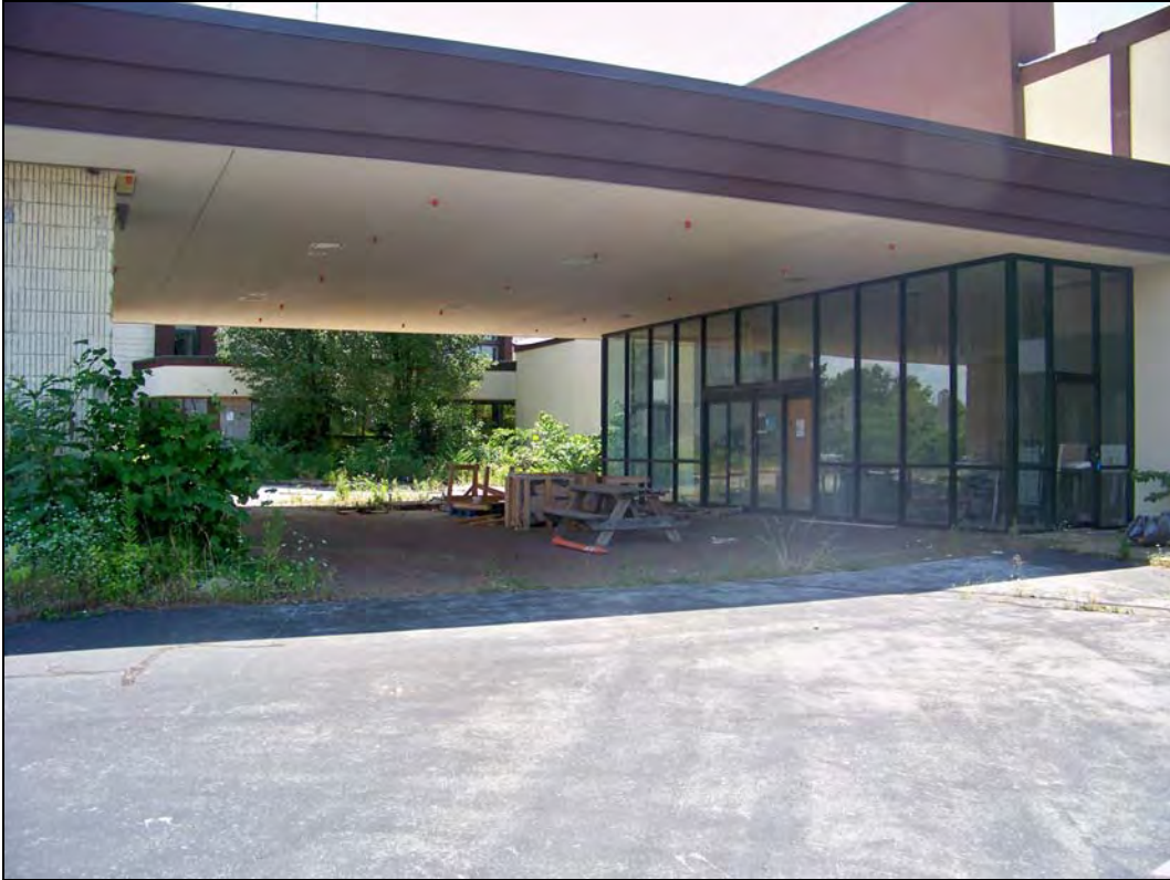
Parcel No. 04-4.0-19-000-000-005.003 – looking east – Joplin Hotel declared “Dangerous Building”
