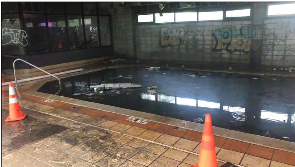
Joplin Hotel – Interior Swimming Pool – Site of fire May 15, 2020 (photo courtesy Joplin Fire Department)
