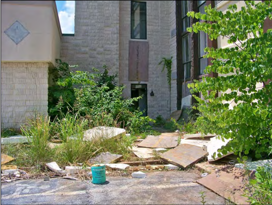
Parcel No. 04-4.0-19-000-000-005.003 – looking south – trash/debris; overgrown vegetation; open door to vacant building
