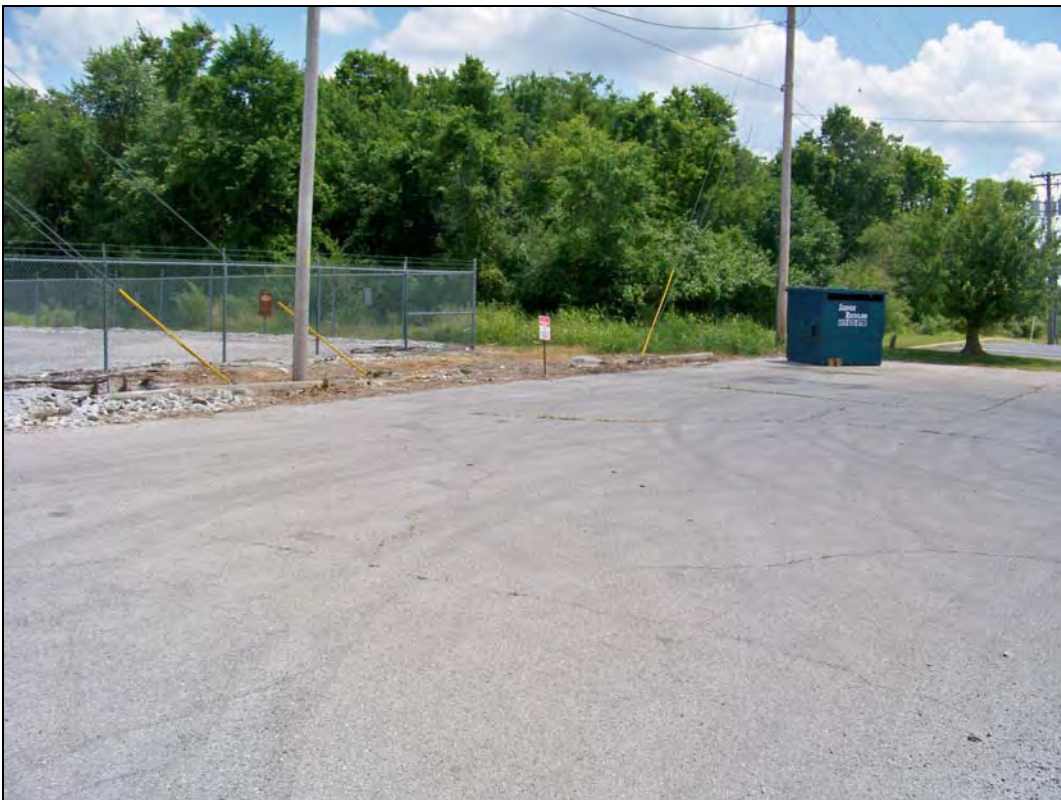
3209 S. Range Line Road – looking southeast – deterioration of pavement; unenclosed trash area
