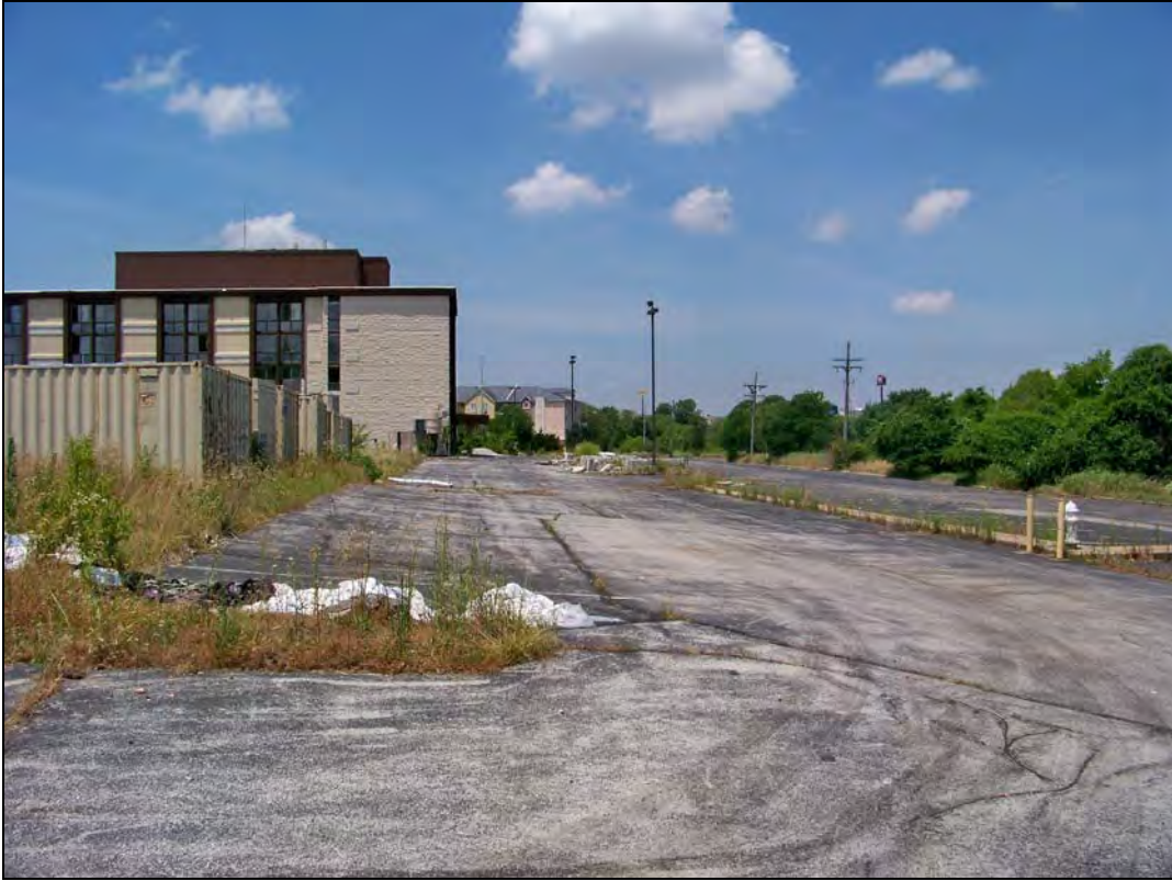
Parcel No. 04-4.0-19-000-000-005.003 – looking west – deterioration of pavement; trash/debris
