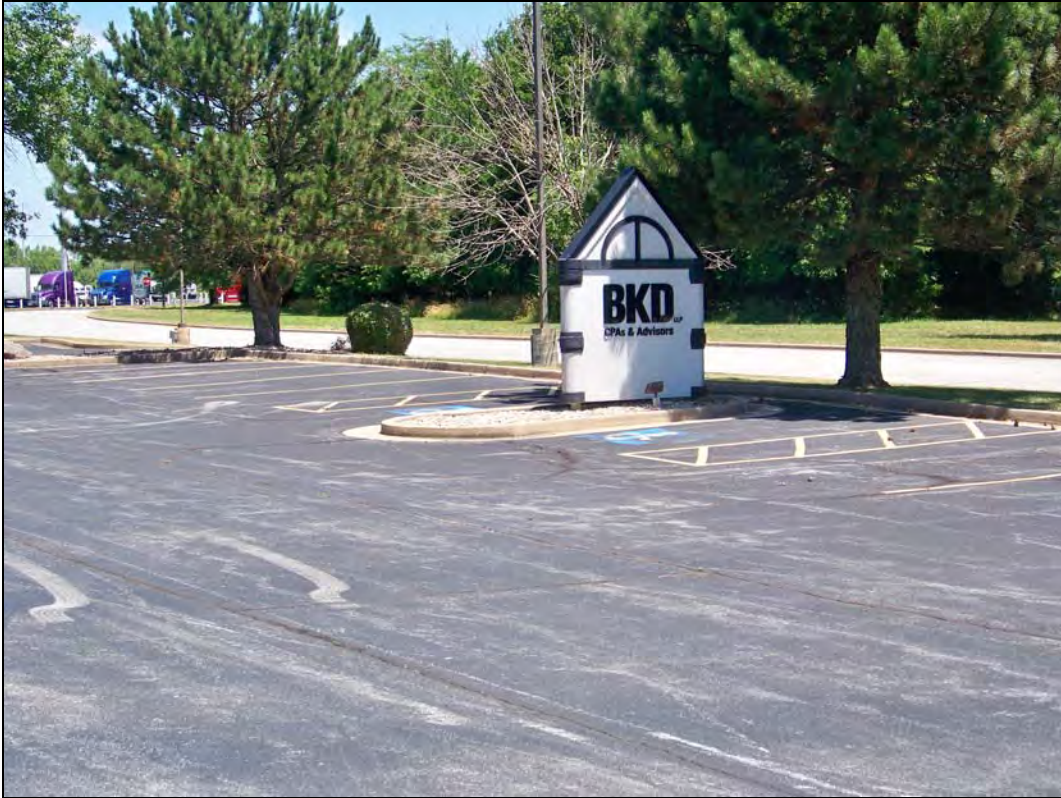
3232 S. Hammons Blvd – looking northeast – lack of ADA signage; ADA spaces located away from front entrance
