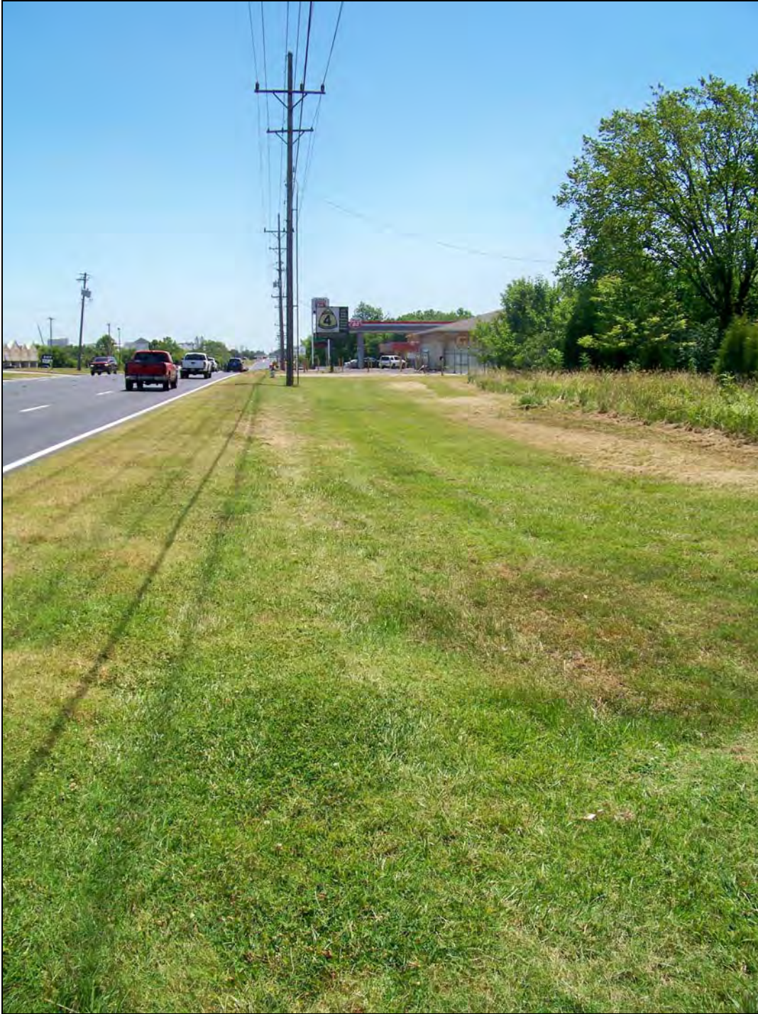
E. 32 nd Street – looking east – lack of pedestrian circulation; lack of curb/drainage ditch
