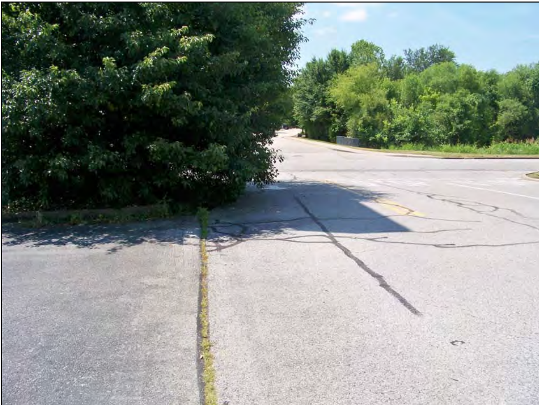
Parcel No. 04-4.0-19-000-000-005.007 – looking south – overgrown vegetation blocking vehicular entrance
