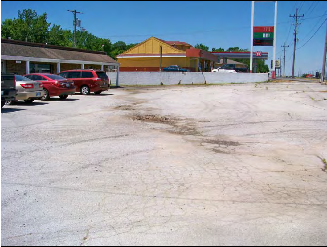
Parcel No. 04-4.0-19-000-000-006.000 – looking west – deterioration of pavement
