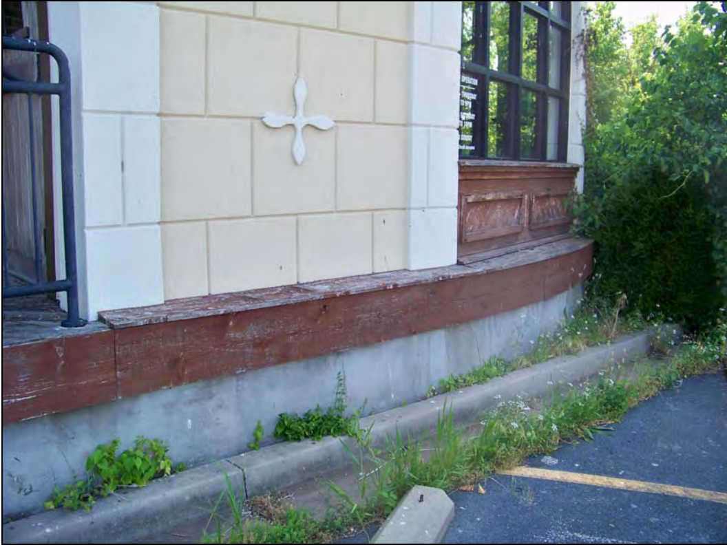
Parcel No. 04-4.0-19-000-000-005.007 – looking southeast – failure of finishes
