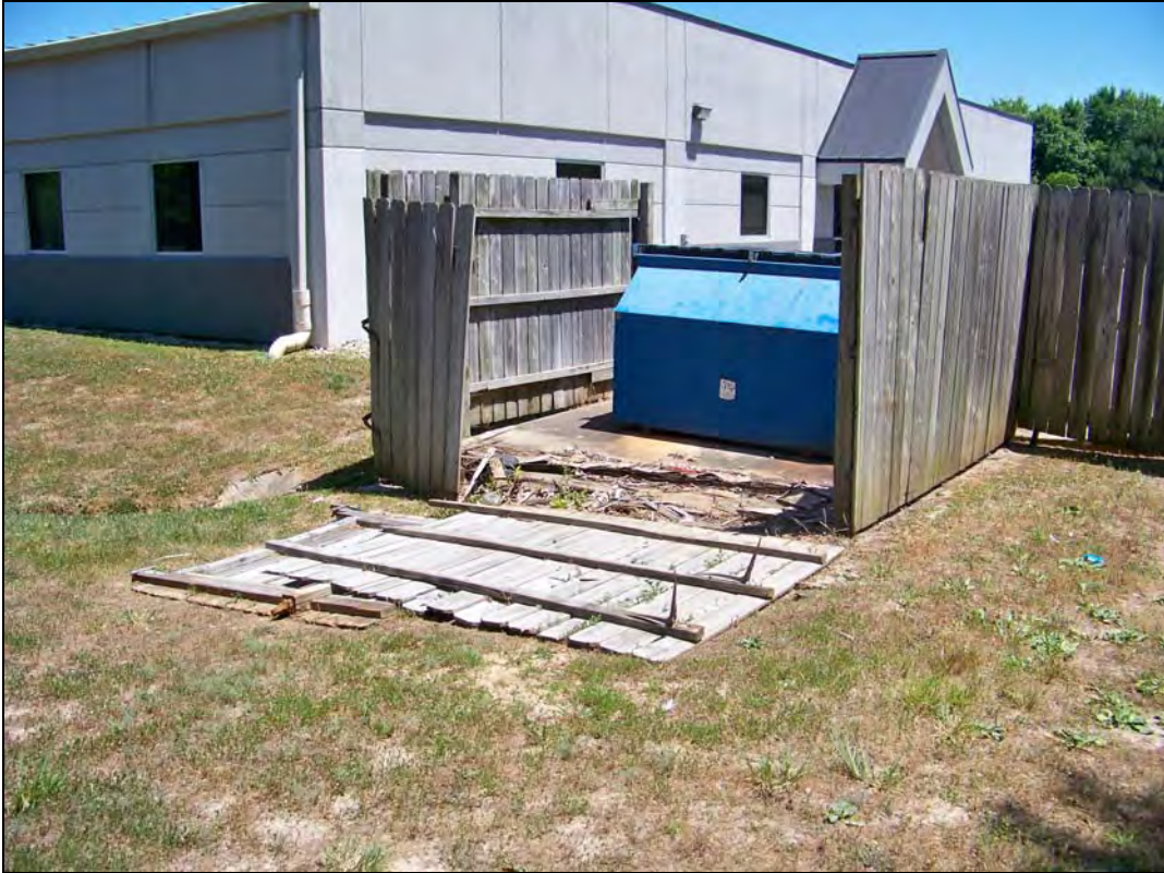
3232 S. Hammons Blvd – looking northeast - deterioration of trash enclosure
