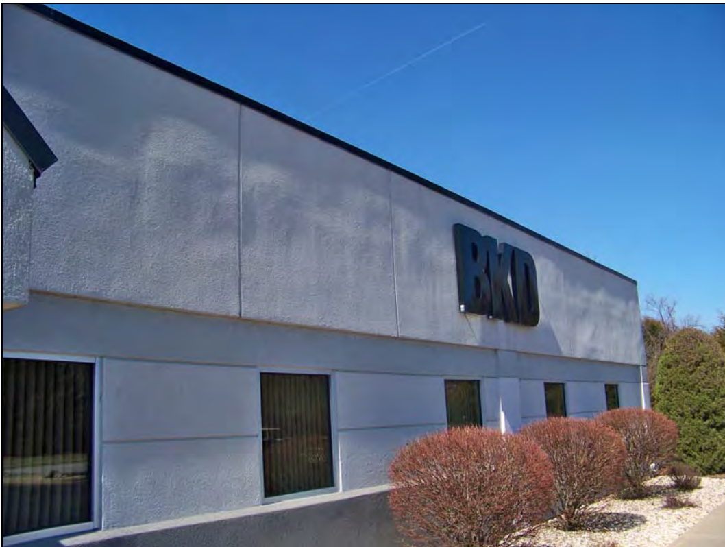
3232 S. Hammons Blvd – looking northwest - deterioration of stucco/EIFS
