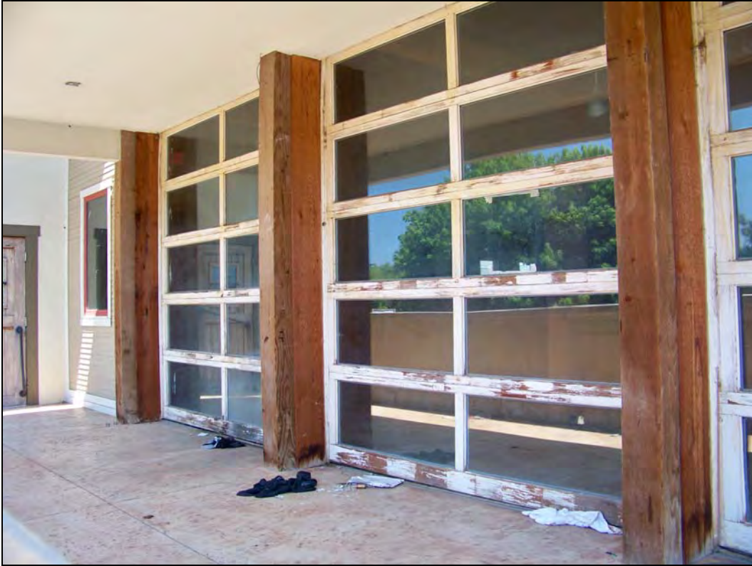
Parcel No. 04-4.0-19-000-000-005.007 – looking north – evidence of vagrant activity; failure of finishes
