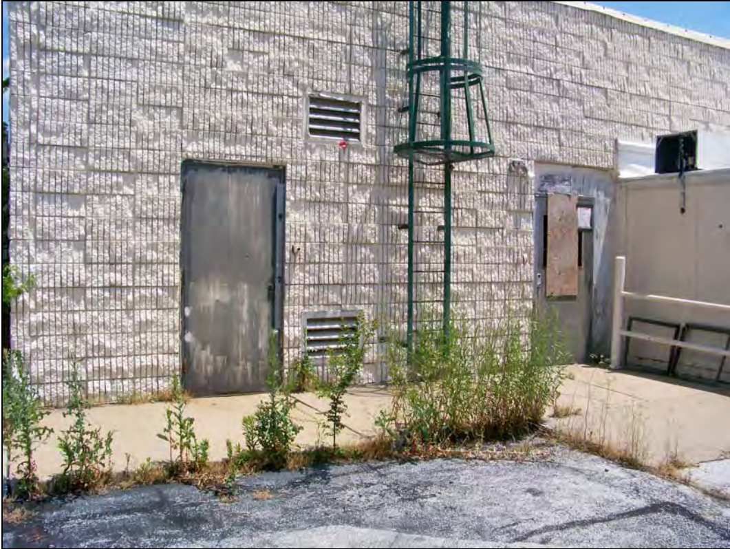
Parcel No. 04-4.0-19-000-000-005.003 – looking north – deterioration of doors; pavement
