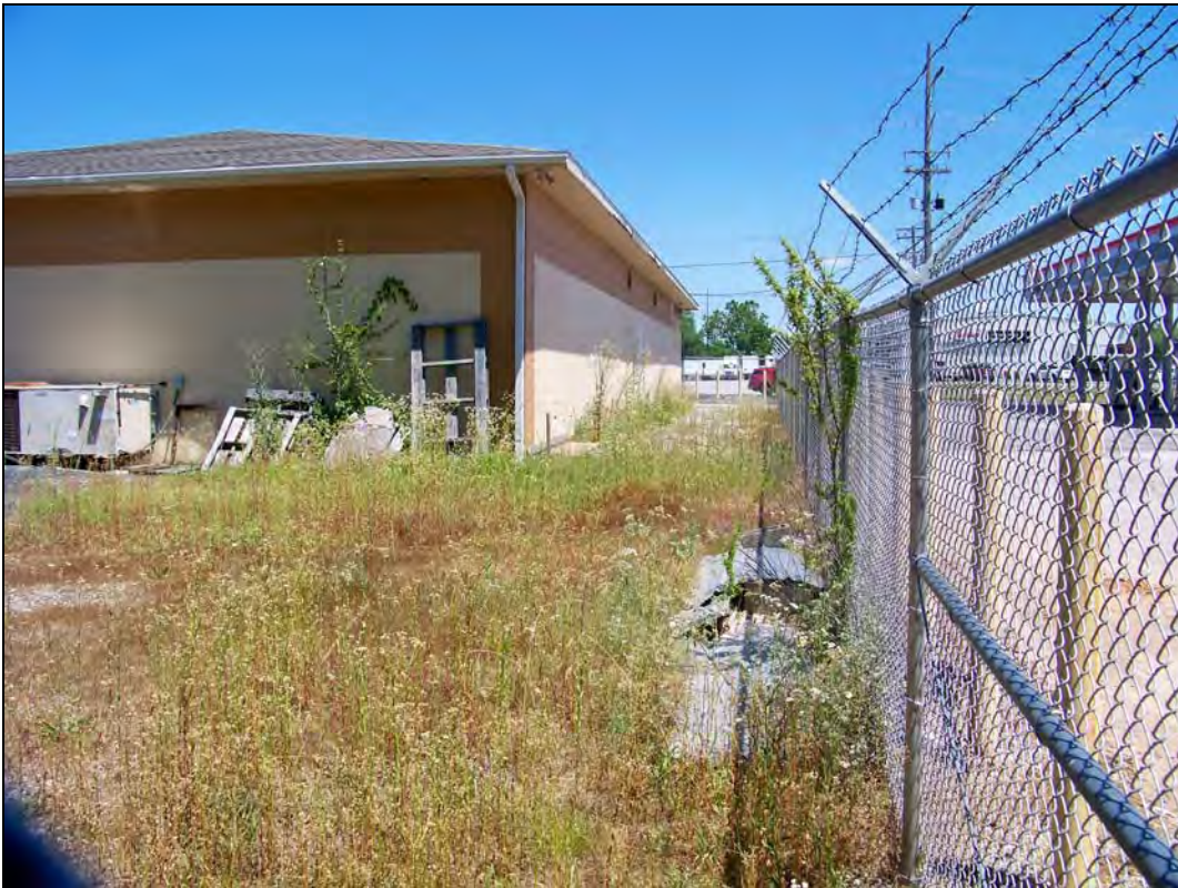
3232 E. 32 nd St – looking north – deterioration of fascia; trash/debris; overgrown vegetation
