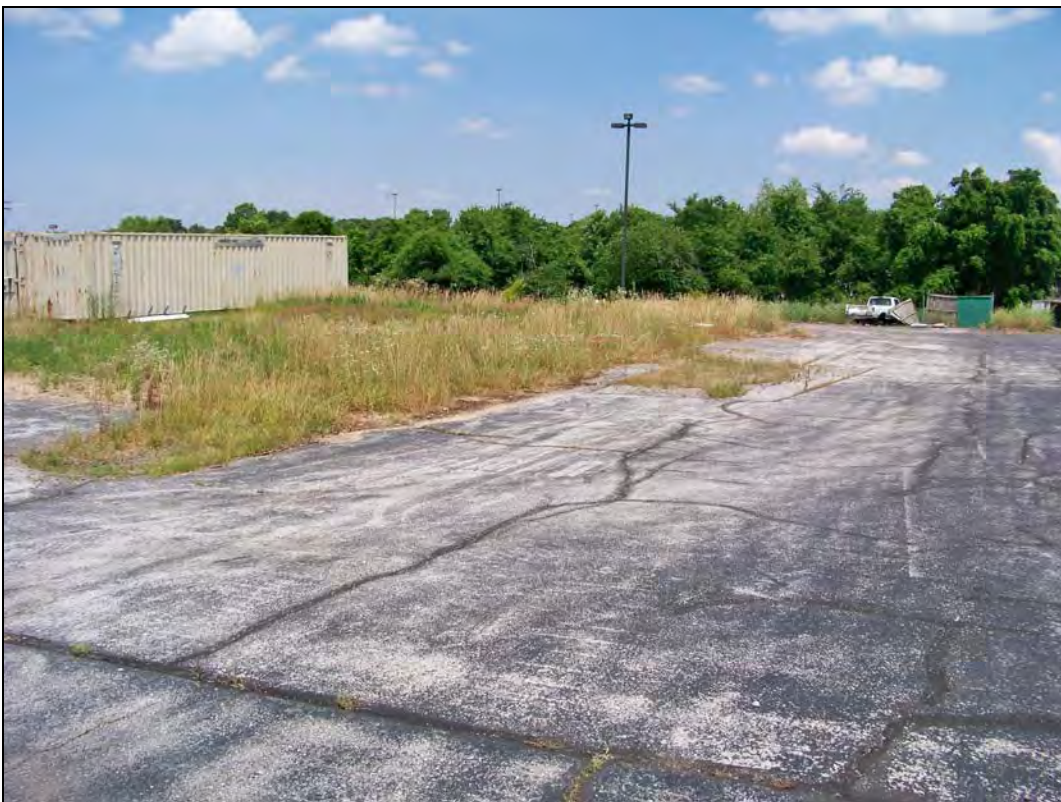
Parcel No. 04-4.0-19-000-000-005.003 – looking north – deterioration of pavement; overgrown vegetation
