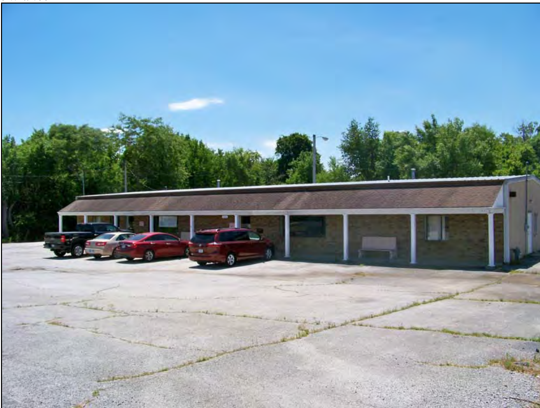
Parcel No. 04-4.0-19-000-000-006.000 – looking south – noncompliance with ADA code (stalls, signage)
