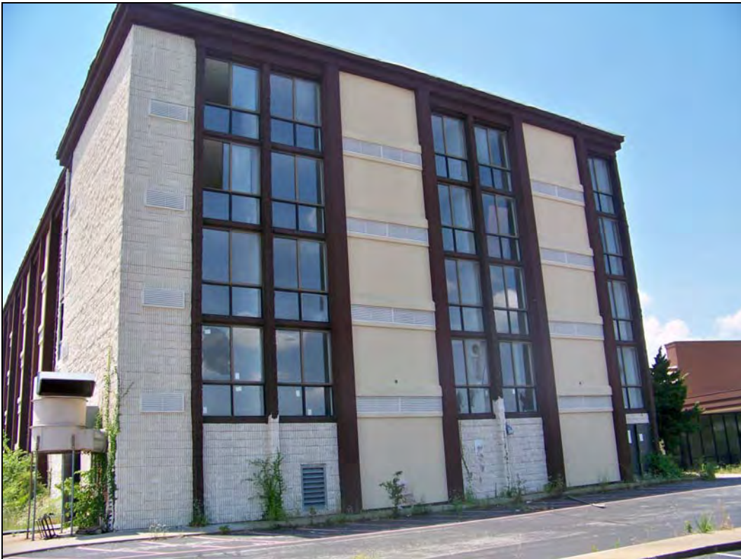
Parcel No. 04-4.0-19-000-000-005.003 – looking south – broken windows; vandalism; overgrown vegetation; open doors to vacant building
