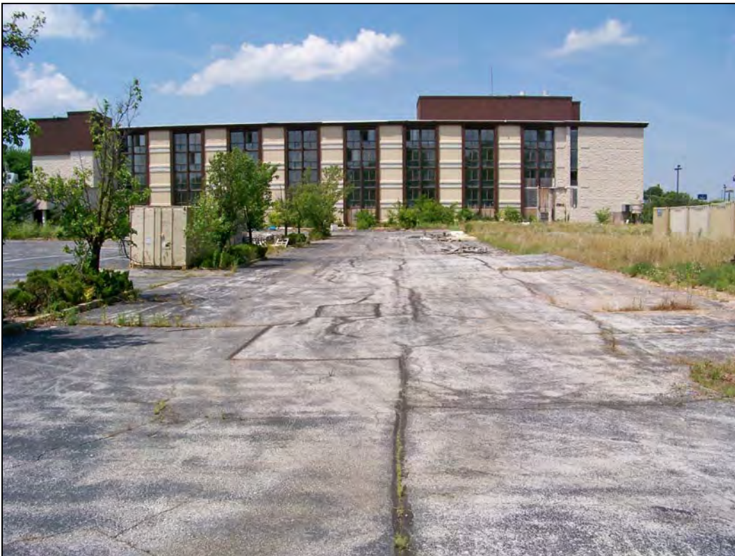
Parcel No. 04-4.0-19-000-000-005.003 – looking west – roof not attached completely; broken windows, doors
