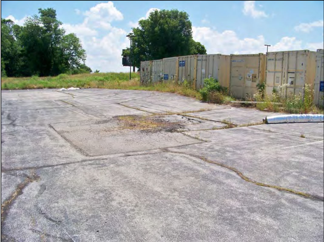
Parcel No. 04-4.0-19-000-000-005.003 – looking southeast – deterioration of pavement; trash/debris
