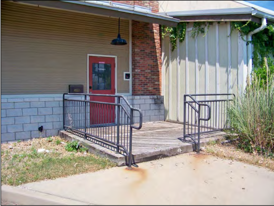
Parcel No. 04-4.0-19-000-000-005.007 – looking northwest – deterioration of deck; failure of finishes
