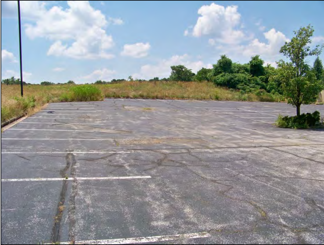
Parcel No. 04-4.0-19-000-000-005.003 – looking south – deterioration of pavement
