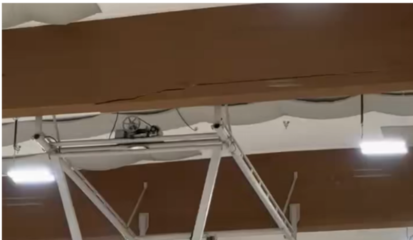
Figure 1 – Beam A Initial Failure
