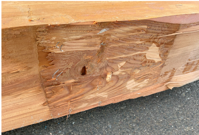
Figure 5 – Failed Scarf Joint
