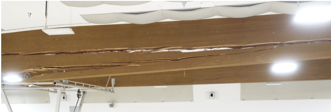
Figure 2 – Beam B Crack
