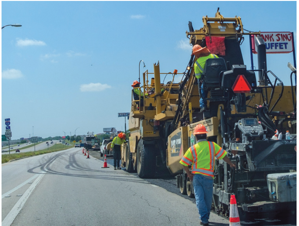
Construction crews work to pave sections of the Interstate 14 frontage road near the Killeen Mall.
