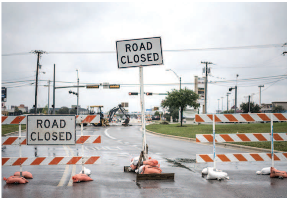
Trimmier Road is under construction from Jasper Drive to Elms Road to widen the north-south thoroughfare in Killeen.
