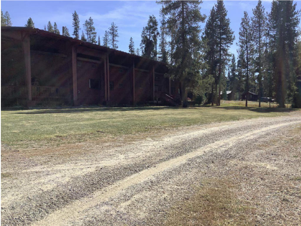
Photo 7. Looking at the existing lodge, which has a protective structure built over it due to a failing roof. In the foreground is the existing road, and disturbed grassland (10/3/2023).
