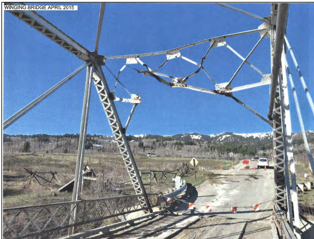
Figure 16. In April 2015, a large truck damaged the west span. It was repaired and opened for traffic in September 2015. (courtesy of Teton County Board of County Commissioners, Staff Report, 1/15/19)
