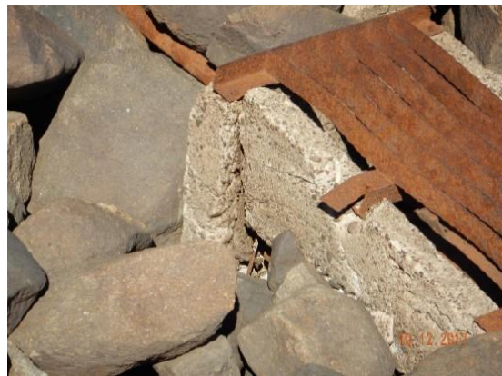
Photo 3. Damaged outlet works inlet structure.
