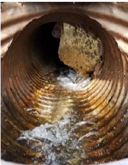
Photo 2. Damaged corrugated metal pipe.
