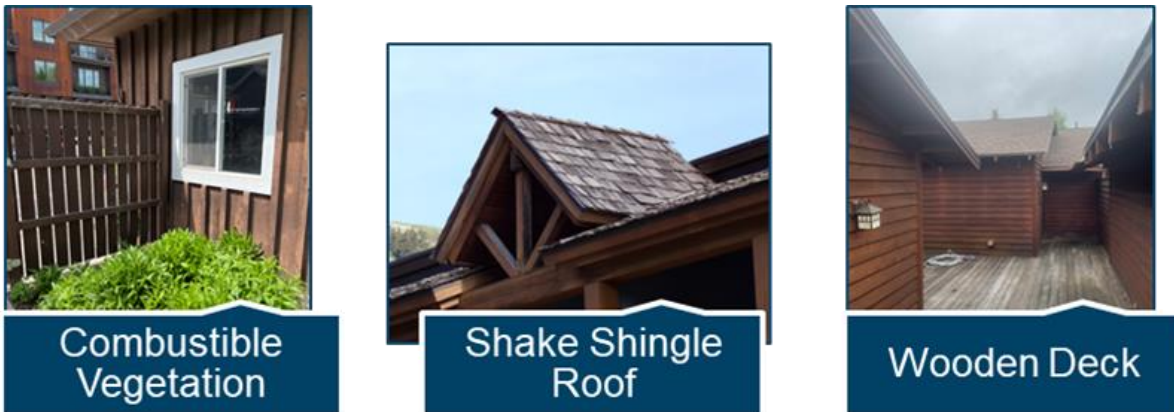
Figure 59: Structure Vulnerability Examples
