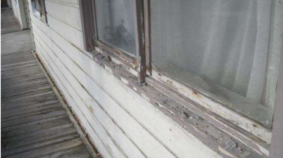
Views of some of the deferred maintenance
