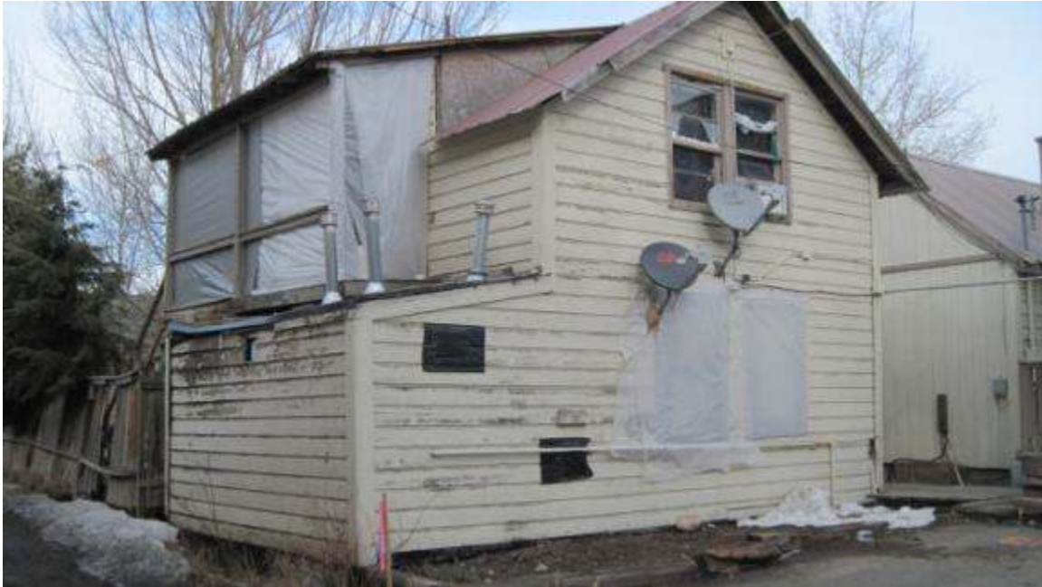
A view of the rear of the improvement and the deferred maintenance
