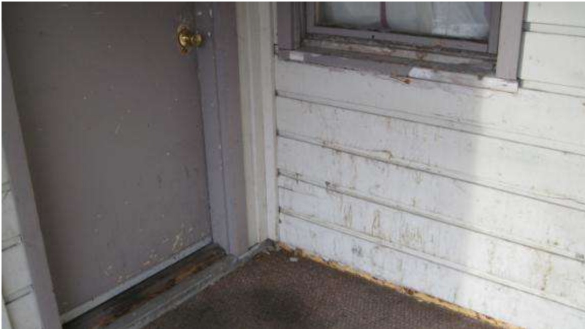
More views of deferred maintenance.
