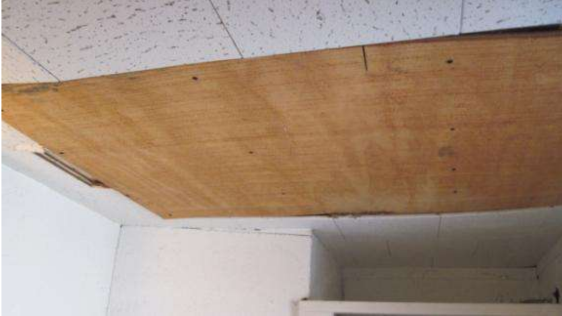
A view of some interior deferred maintenance.
