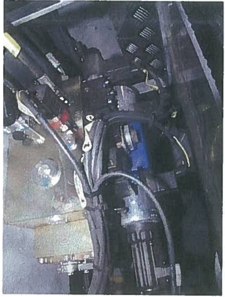
Siemens 2.3 Hydraulic Manifold (similar to a car's brake master cylinder)
