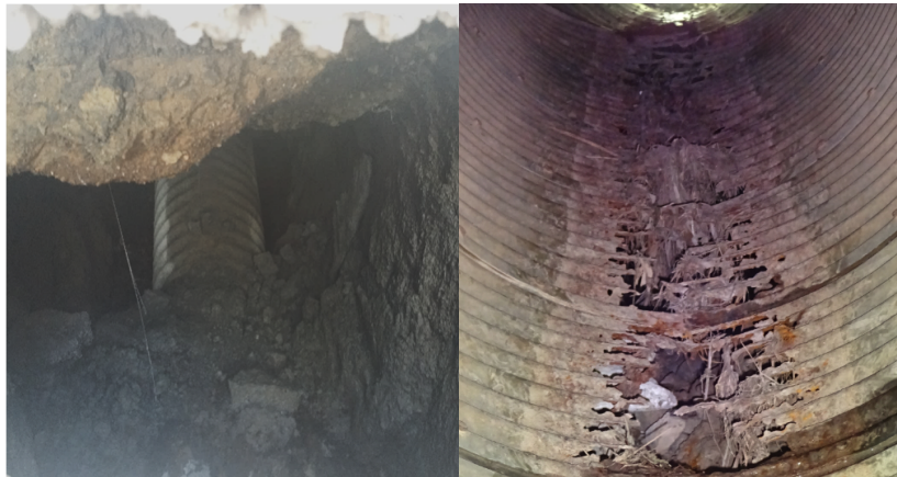
Figure 1. The GIS Data Collection process will include documentation of defects and identification of critical infrastructure. The above pictures are from a previous Snyder and Associates project.
