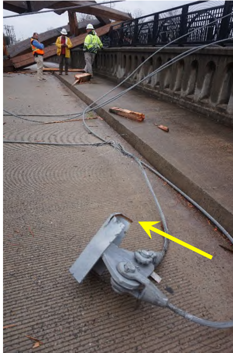
Photograph 21) – Another view of S15. The part in Photo 14 detached from this end.
