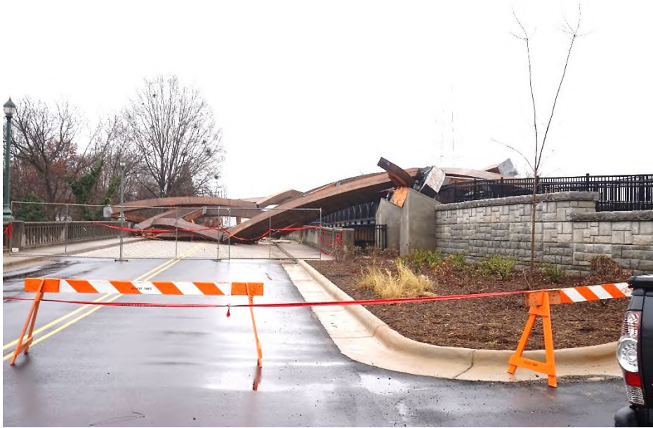
Photograph 1) – Overview of collapse taken from west end of Main Avenue bridge.
