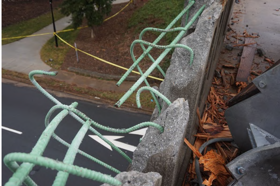
Photograph 30) – Damage to the concrete guardrail system on the Main Avenue bridge.
