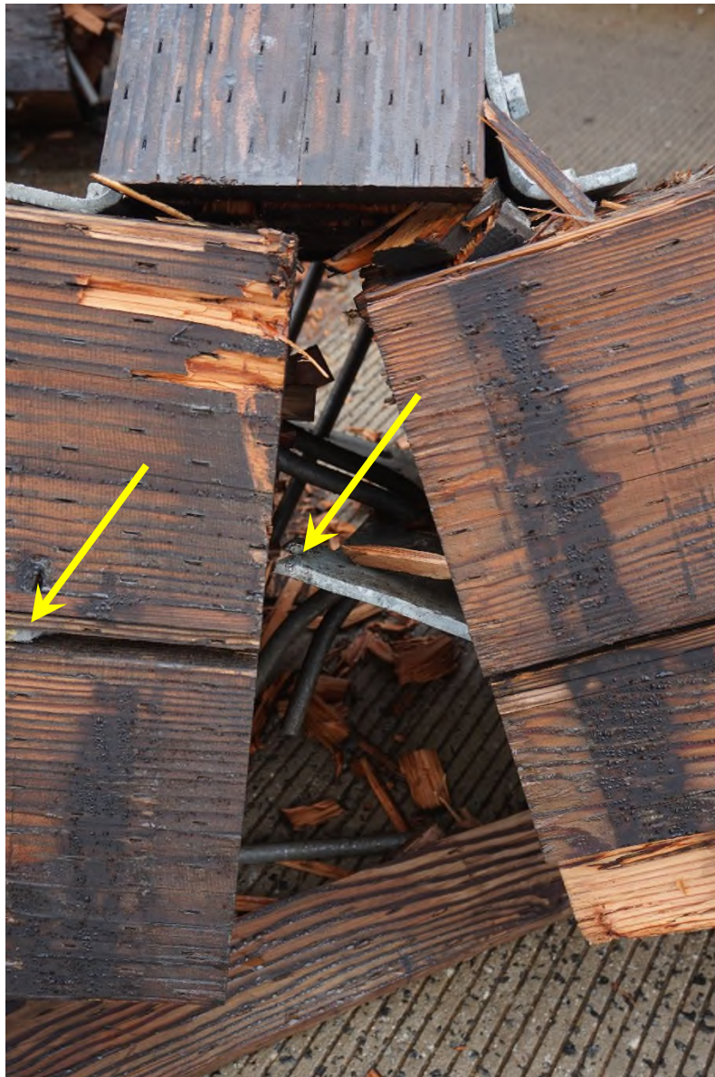
Photograph 29) – Failure of the kerf plate at a connection.
