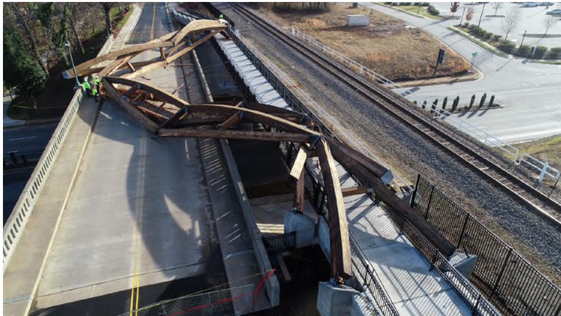
The collapsed Arches and all three bridges. (Credit: from Neill's files – image DJI_0039)
