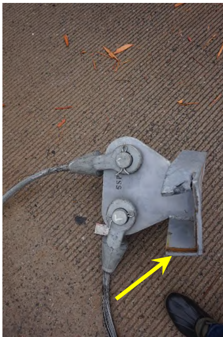
Photograph 20) – Part S15. The piece circled in Photo 14 detached from the end of this Part.
