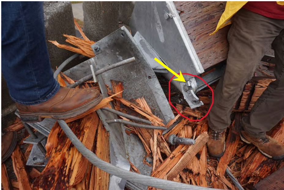
Photograph 14) – Circled in red is part of Mark S15. Welds failed and this part detached from the part shown in Photo 13.
