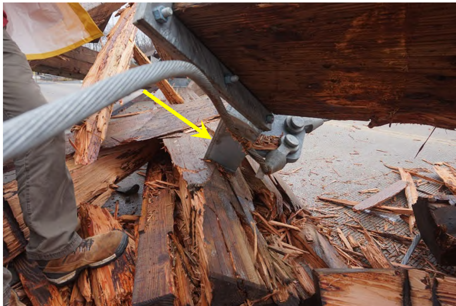
Photograph 15) – View of the intact steel cable bracket, which partially detached from the connection.
