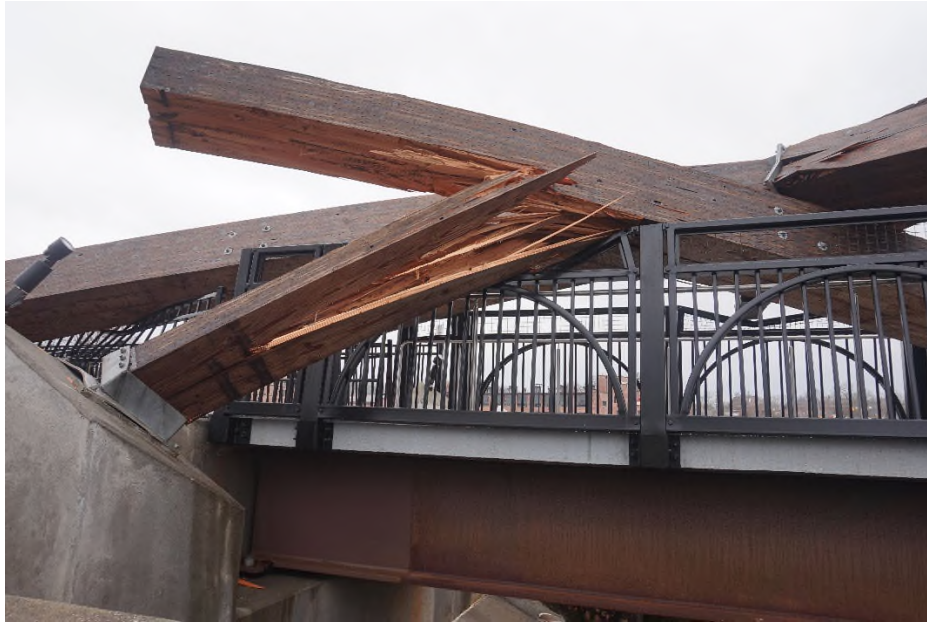
Photograph 7) – The lower arch base connection at the east end. The steel “shoe” pulled off of the base plate. The GluLam member splintered.
