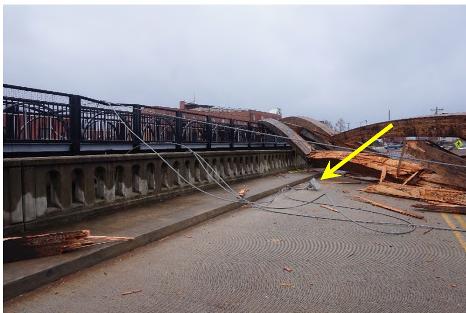
Photograph 18) – Part S15. This would have been connected to the lower part of the arch. It pulled apart from the piece shown in Photo 14.
