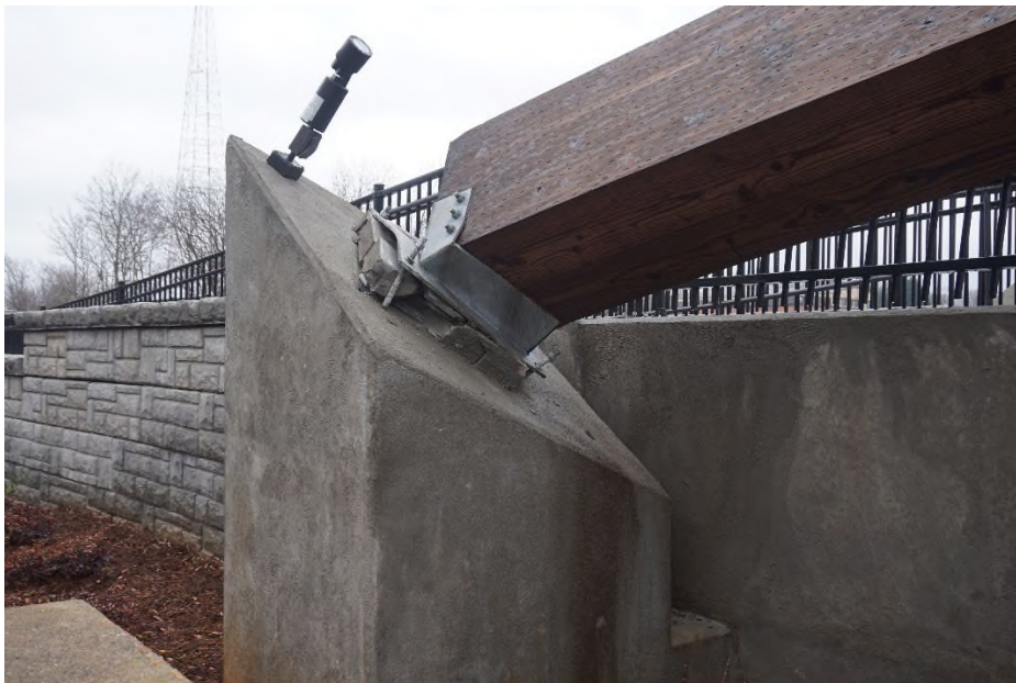
Photograph 8) – The upper arch base connection at the east end. The steel “shoe” pulled off of the base plate and base plate yielded.
