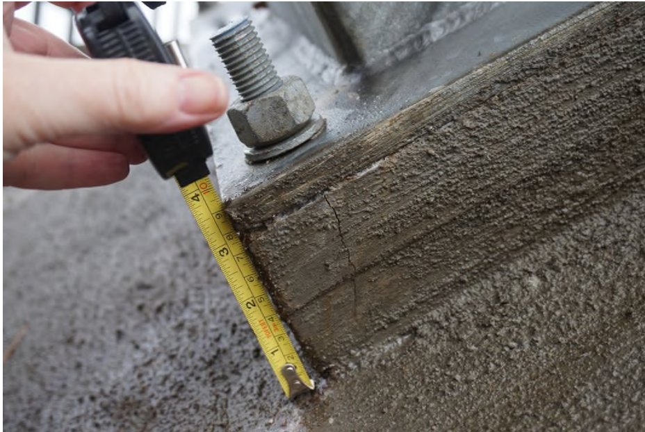
Photograph 5) – Grout below base plate at NW base connection is 3” thick. There were also steel bearing plates within. Each base plate had four \frac{3}{4} ” diameter anchor bolts.
