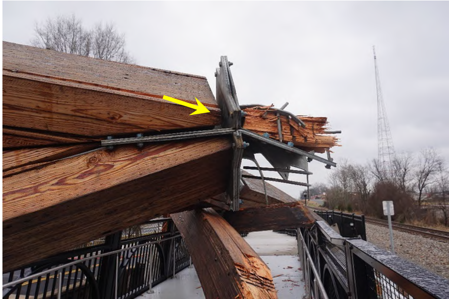
Photograph 24) – The connection of node 4 (or 22 which is identical). From the security videos we see that the arch began to pivot and fall over at this node.
