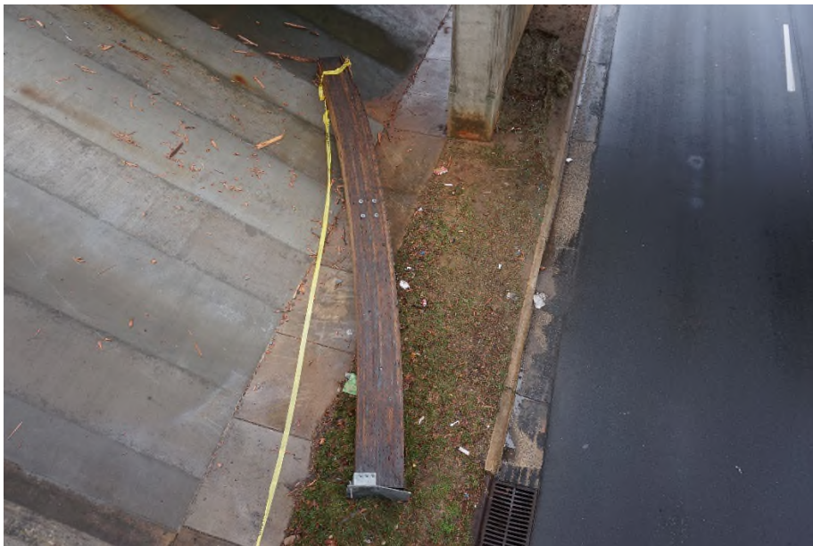
Photograph 31) – Debris landed below on NC Hwy 127.
