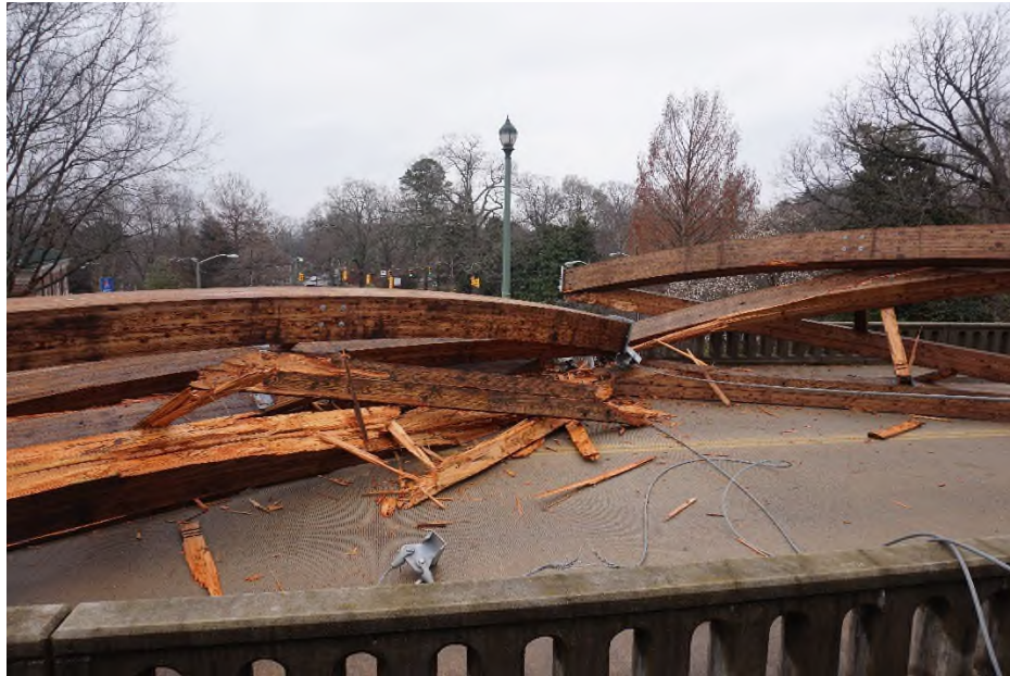
Photograph 23) – Overview of the top node of the arch. The upper and lower arch connected at node 13. The two sets of dual cables connected to the bottom arch and also to the upper arch.
