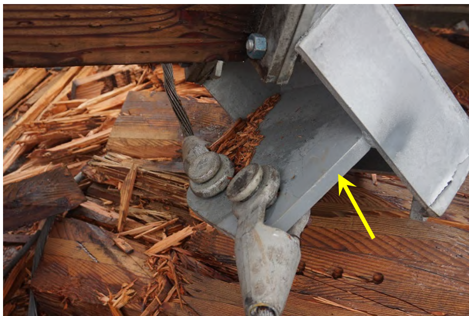
Photograph 16) –The intact cable bracket.
