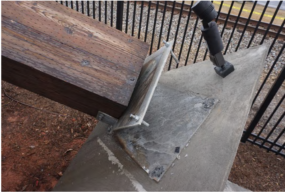
Photograph 11) – Southwest base connection. Anchor bolts pulled out.
