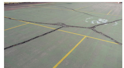
At Vint Hill Village Green, cracked courts need resurfacing.
