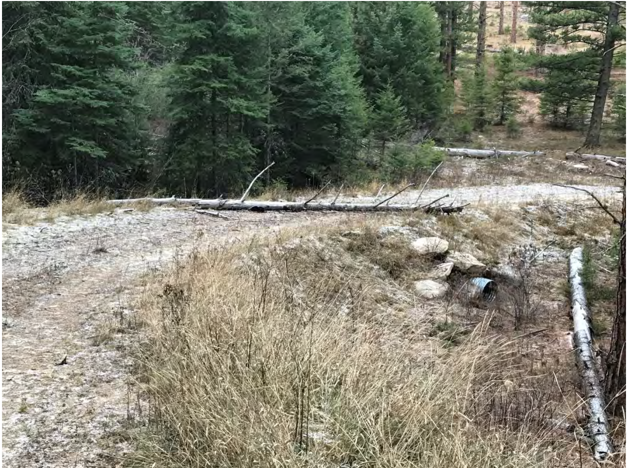
12-1-2023 photo of the road to unit 2c showing that culverts have not been removed and the road has not been scarified, reseeded, or put into storage. A Coyote Coulee trail crossing is just out of view to the right.
