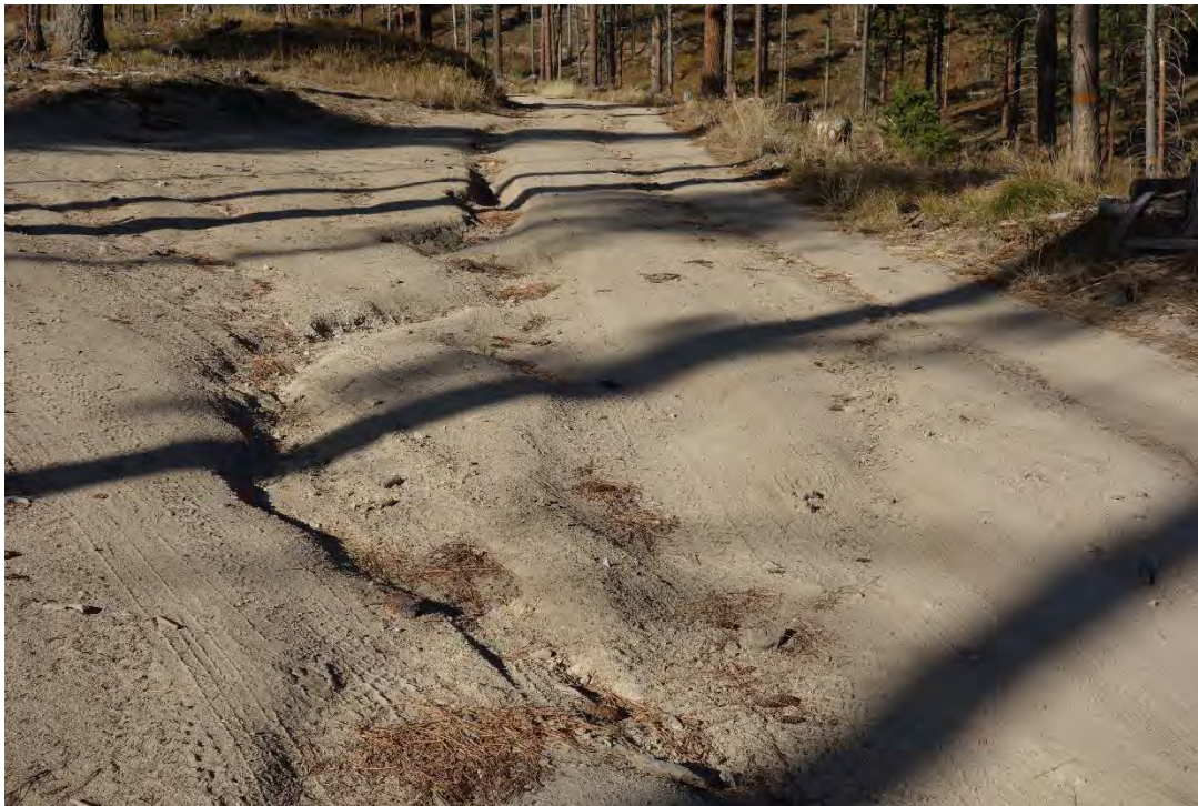
10-3-2022 photo of the new intersection of FR 496 and FR 5620. Current situation (3-2024) is the same or worse. Water flows down the road for ¼ mile before dumping into an intermittent tributary of Moose Creek.
