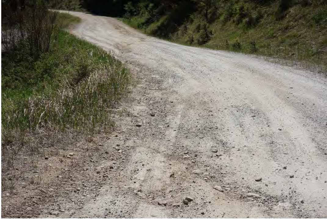
5-17-2022 photo of FR 496 just above the Moose Creek crossing at top left. Gullies were dumping sediment directly into Moose Creek at upper left. At the time, re-routing of NFSR 5620 to improve Moose Creek was ongoing.. Later regrading of the road temporarily fixed the situation, but by 3-2024 the gullies were back.
