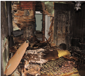
COURTESY PHOTO Fire contained to one bedroom
