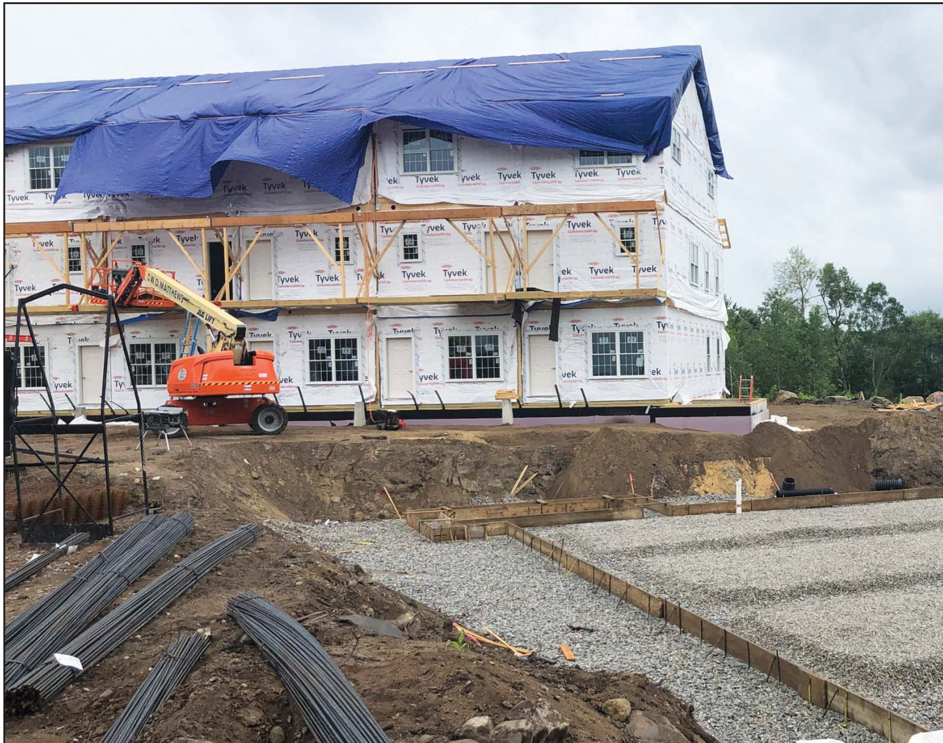
Modular units are being used to construct two buildings of 12 apartments each behind the Whitesides building on Route 16 in North Conway. The 24 one- and two-bedroom apartments will be part of Alpine Place Luxury Apartments being marketed for professionals coming to the Mount Washington Valley, according to Brenda Leavitt of Badger Realty. For story, turn to page 5. (TOM EASTMAN PHOTO)
