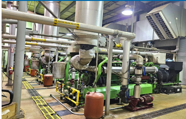
Renewable Energy Generation
