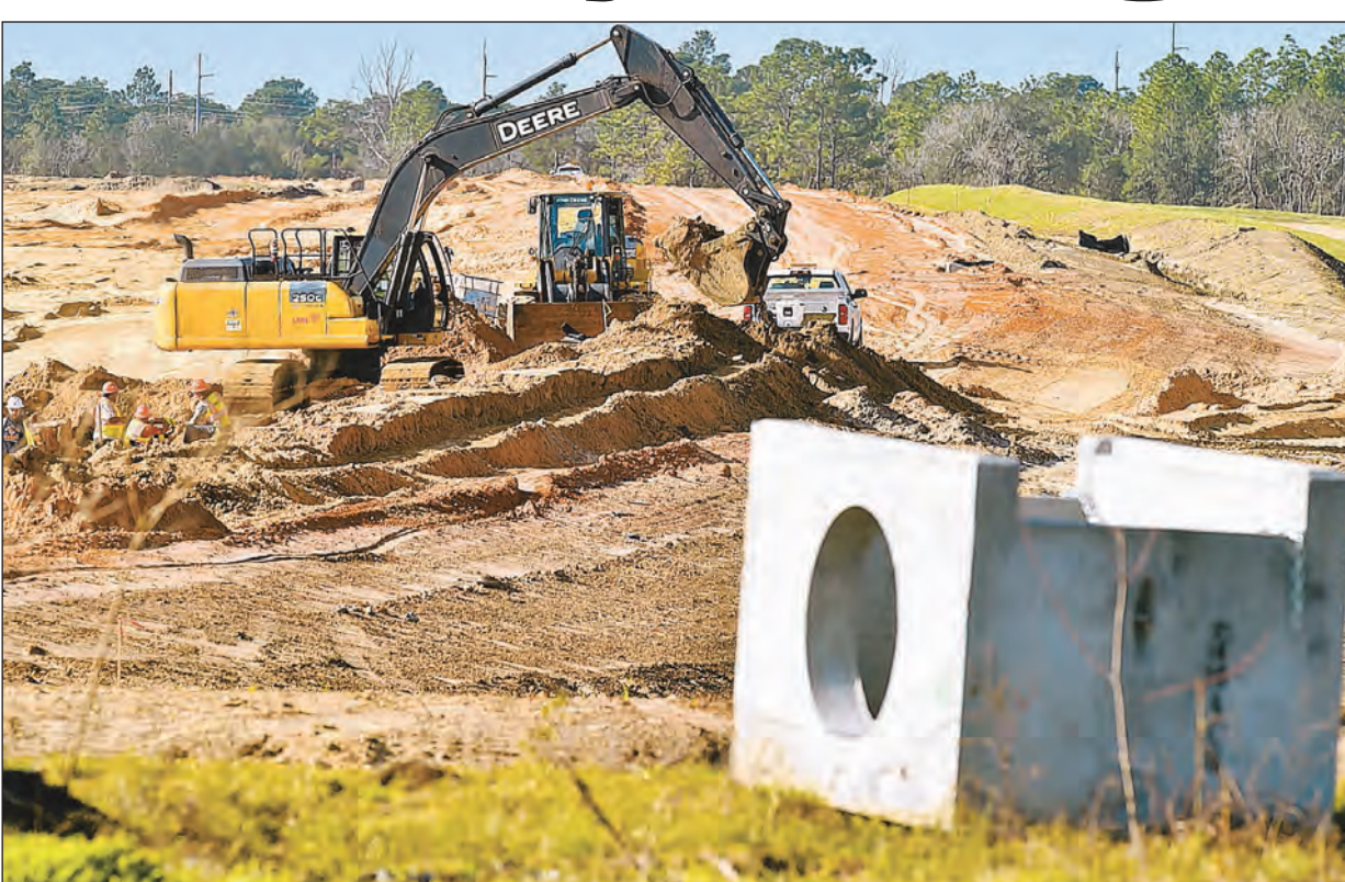
Construction on the Suncoast Parkway continues Monday, Feb. 22, near the intersection of State Road 44 between Lecanto and Crystal River. A state official said plans for an extension of the highway farther north through Citrus County will not be affected due to budget shortfalls.
