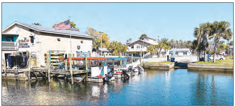
As a result of its King's Bay Riverwalk construction, Crystal River will close the popular, city-owned boat ramp in between Bird's Underwater Dive Center and Charlie's Fish House. The ramp offers access to King's Bay and points west to the Crystal River and Gulf of Mexico. See RAMP/Page A7
