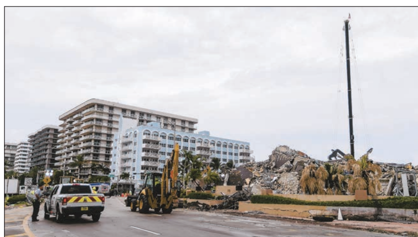
Associated Press Rubble and debris of the Champlain Towers South condo can be seen in Surfside, Tuesday. The rubble shown here is from the front portion of the condo towers, which was demolished 11 days after the back part of the tower collapsed with people inside.
