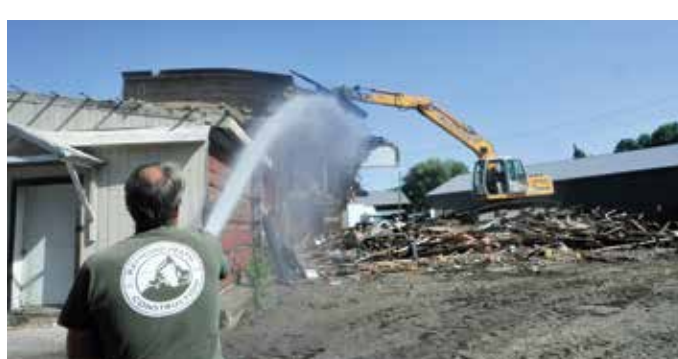
Andy Heath, of Raymond Heath Construction, focuses a water hose on the former KC Rentals building on Bay Street in St. Johnsbury on Monday, Aug. 26, 2019, while Dan Heath works an excavator to tear down the building. The water was used to keep the dust down from the demolition. (File Photo by Dana Gray)
