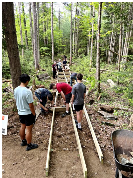
Members of Littleton High School's Project Bike Tech class rebuild a 60-foot long bridge at PRKR MTN trails in Littleton, N.H. (Courtesy Photo)
