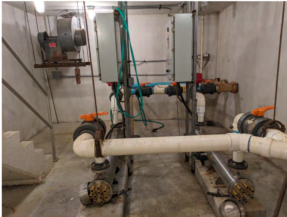
Figure 2-10: UV Disinfection Systems & Control Panels
