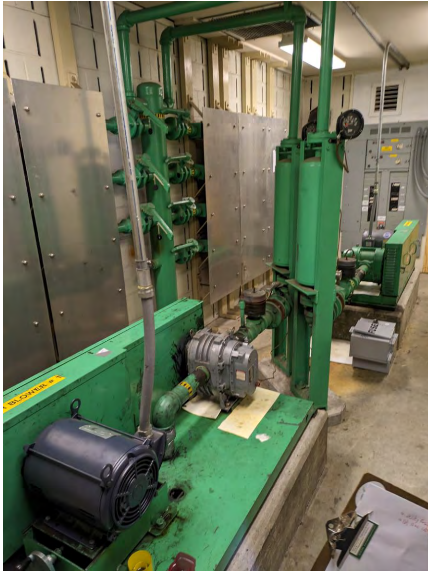
Figure 2-9: Aeration Blowers & Discharge Manifold
