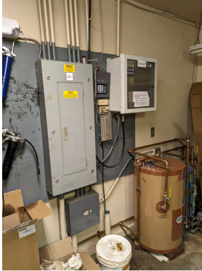
Figure 2-12: Electrical Service & Water Heater
