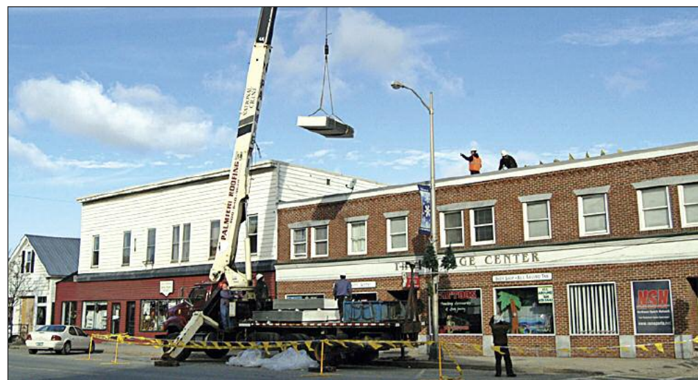
Palmieri Roofing at work in Lyndonville. The company has been topping off area structures for the past 25 years.
