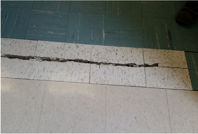
Patched asbestos tile
