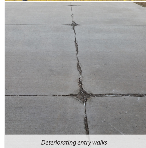
Deteriorating entry walks
