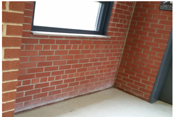
Stained brick walls in corridor
