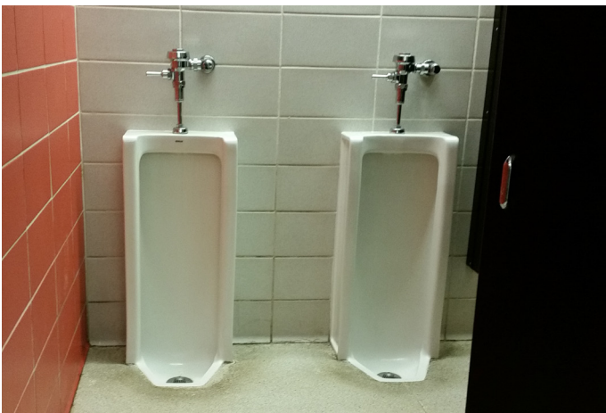
Stained terrazzo and block walls
