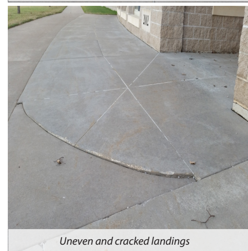
Deteriorating entry walks
