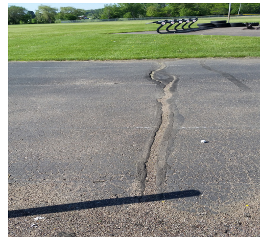
Lateral cracks in track
