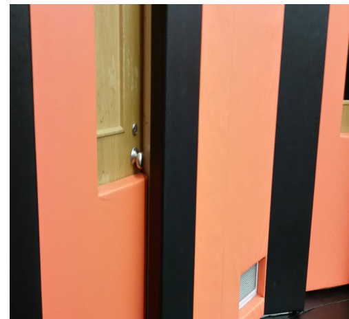
Non-ADA compliant door hardware
