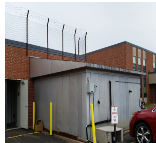
Bump-out refrigeration unit
