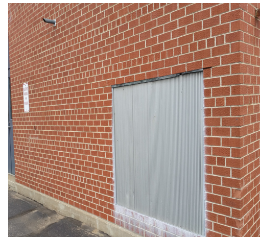
Boiler make-up air intake louver
