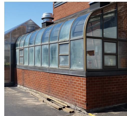
Deteriorating greenhouse wall base
