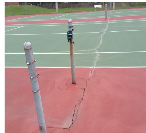
Cracks on tennis courts
