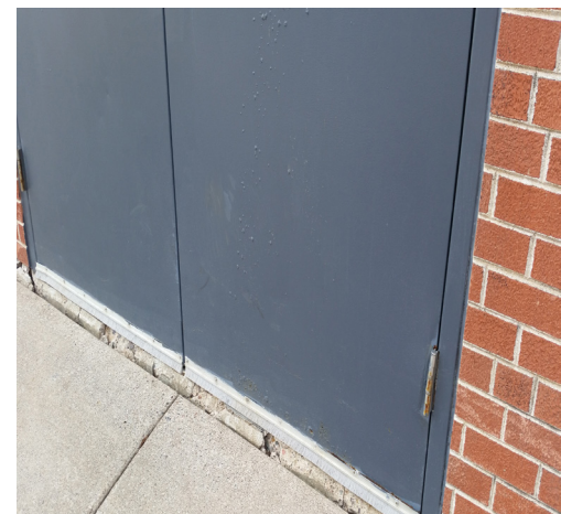
Cracked exit door threshold
