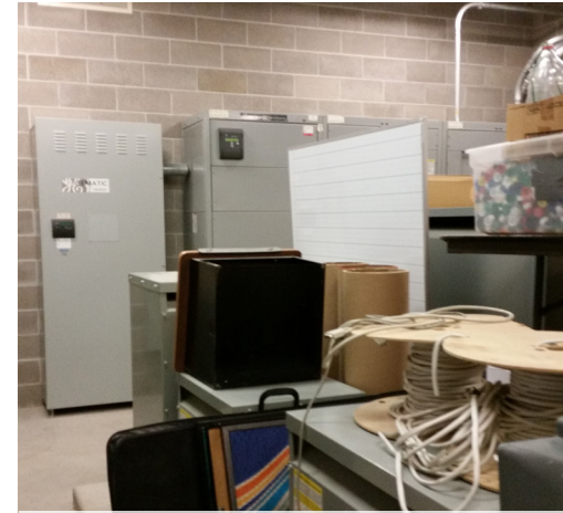
Main electrical room improper storage
