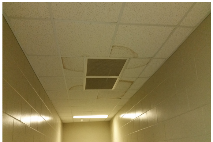
Stained ceiling tiles
