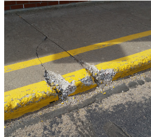
Broken out curbing in front of school
