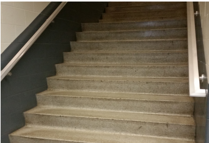
Dingy and stained terrazzo stairs and walls
