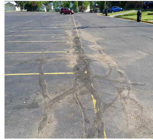
Asphalt cracked, worn, and faded paint
