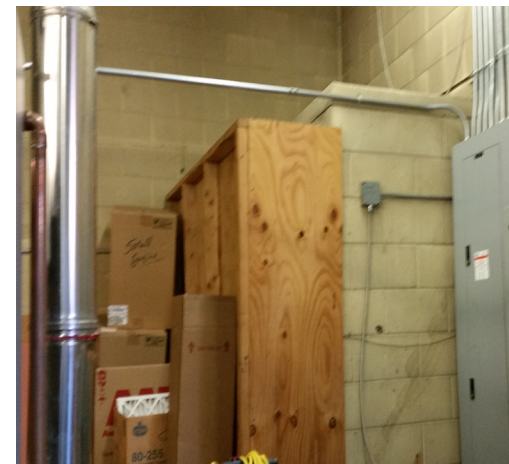
Boiler wood make-up air cover
