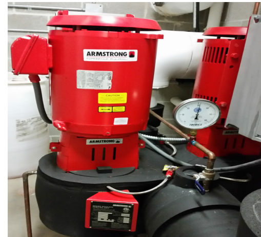
2017 chilled water pump
