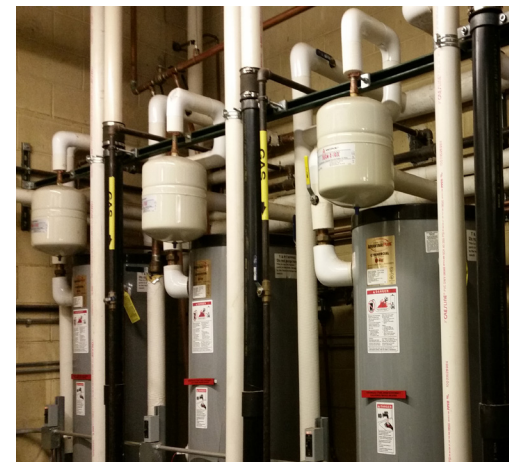
Central domestic water heating
