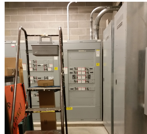
Main electrical room lack of clearance
