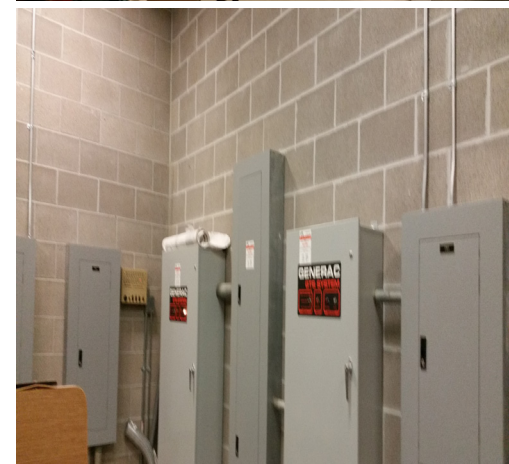
Generator transfer switches
