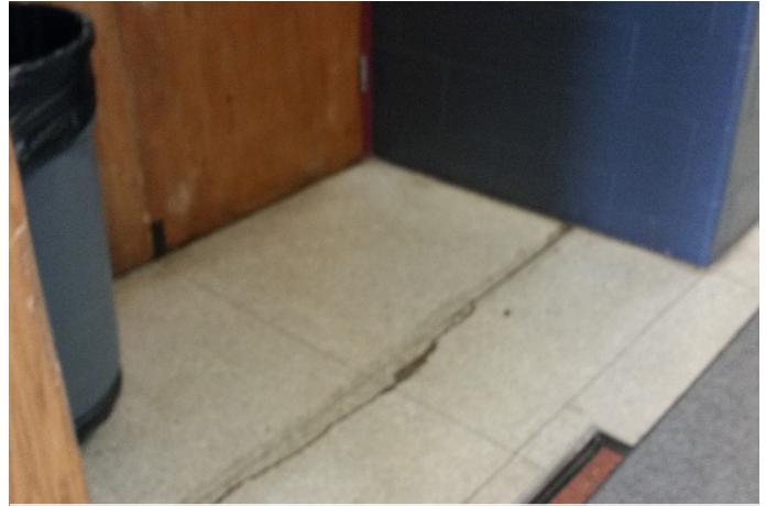
Cracked terrazzo flooring in corridor
