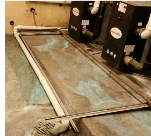
Interior condensate pipe and channels
