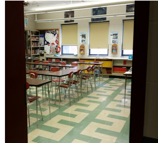
Asbestos tile in classrooms
