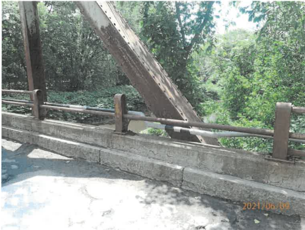
Photo 13: South Railing, 1st and 2nd panel from West Abutment upper rail missing
