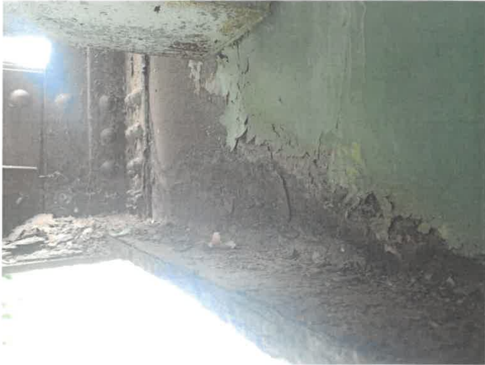
Photo 31: Floorbeam FB5 at south end, east face with rust
