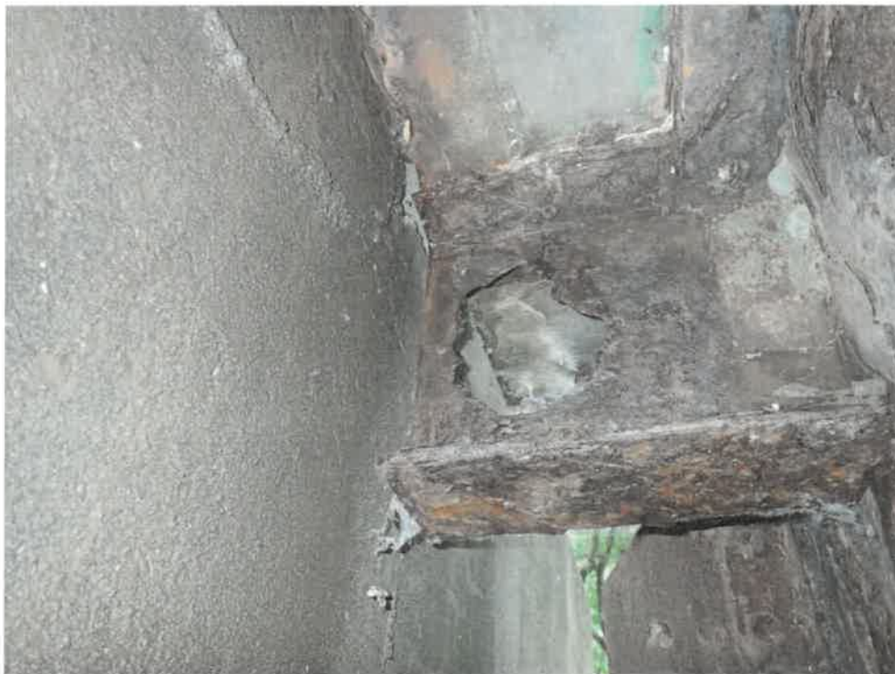
Photo 24: Stringer S5 at Floorbeam FB8 with perforation at end
