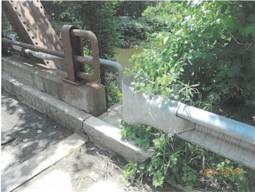
Photo 9: Southwest Approach bridge and approach curb misalignment and missing guardrail transition
