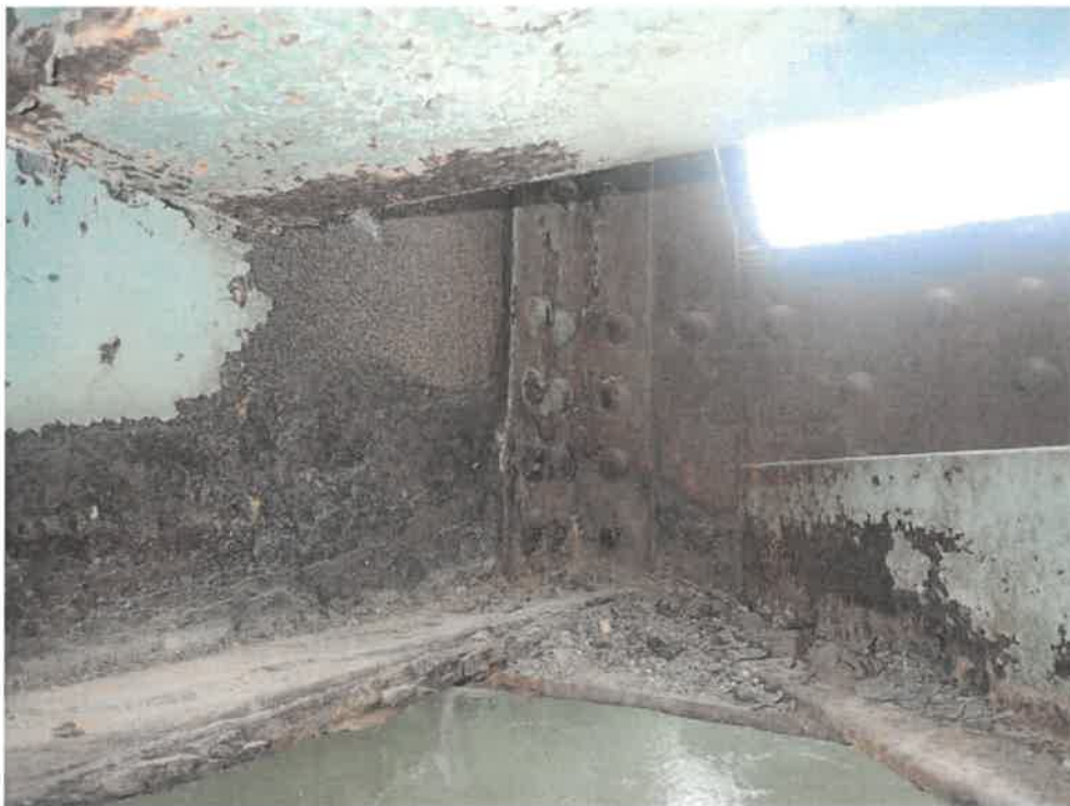
Photo 30: Floorbeam FB5 at north end, east face with heavy rust and section loss
