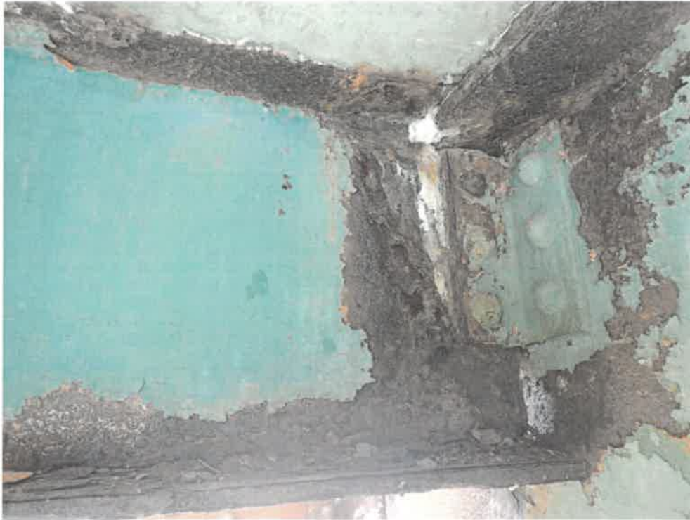
Photo 21: Stringer S5 at Floorbeam FB3, north face with rust and section loss
