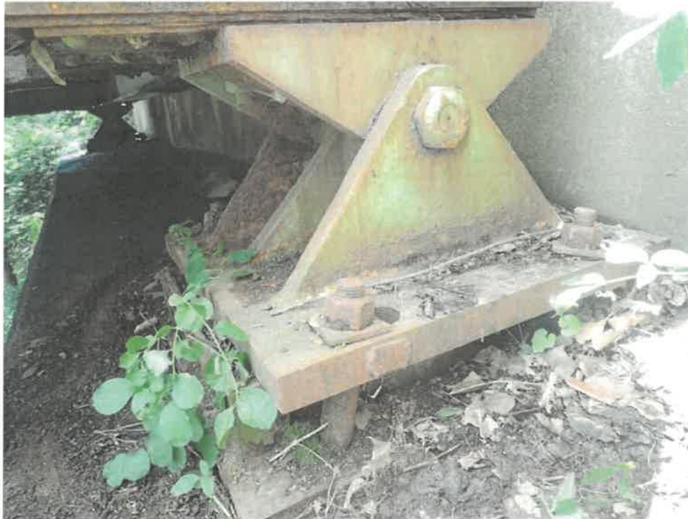
Photo 41: Northwest Bearing with overexpansion and bent anchor rods
