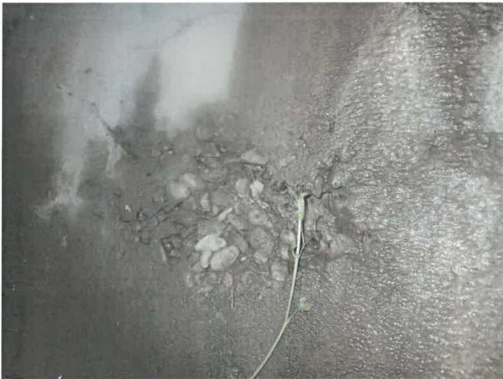
Photo 44: West Abutment south of Stringer S4 with spall
