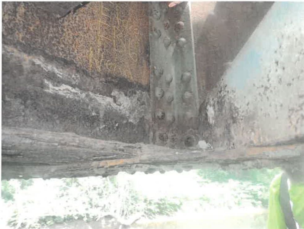
Photo 32: Floorbeam FB6 at north end, east face with heavy rust and section loss
