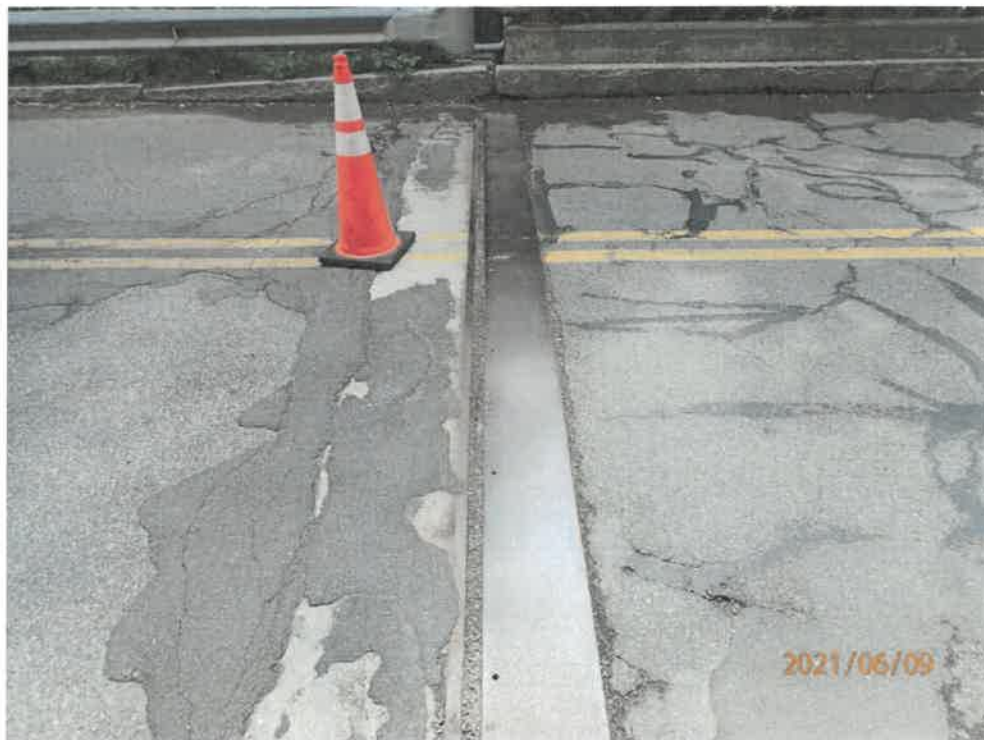
Photo 16: East Abutment deck joint with partially patched header and approach pavement cracked with some break-up
