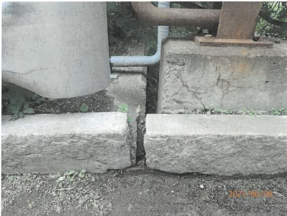
Photo 10: South Curb at East Abutment with gap between bridge and approach curbs
