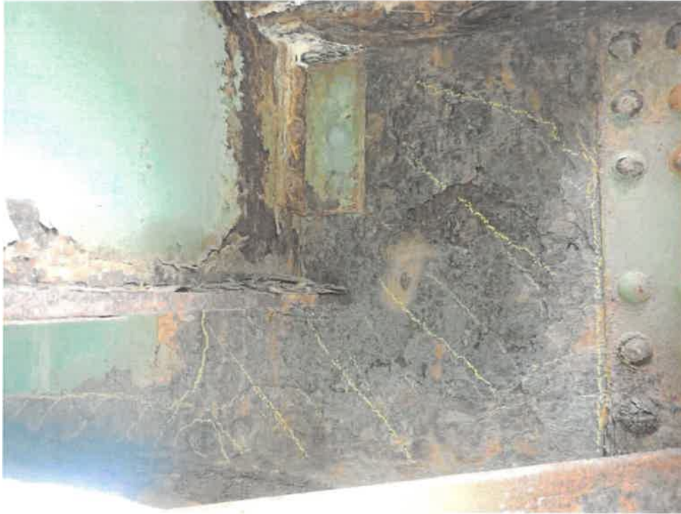
Photo 27: Floorbeam FB2 at south end, west face with heavy rust and section loss
