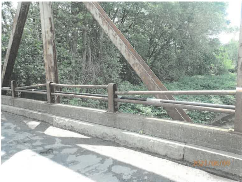
Photo 14: South Railing, 10th and 12th panel from West Abutment upper rail disconnected
