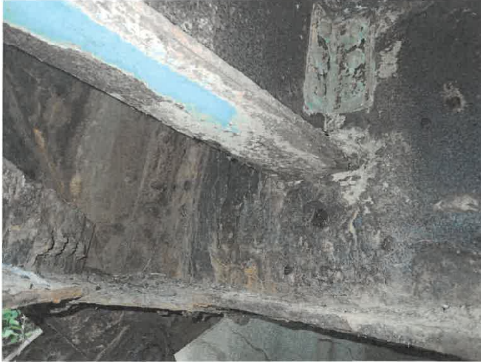
Photo 25: Floorbeam FB0 at Southwest Bearing, east face with heavy rust, perforations, and section loss
