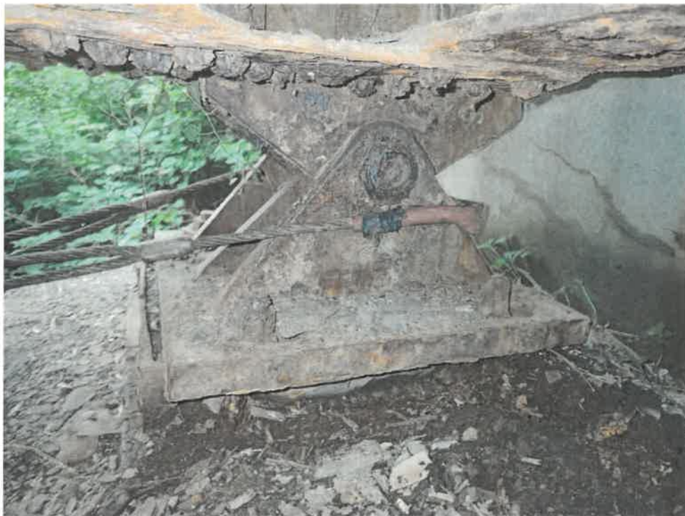
Photo 42: Southwest Bearing with debris, rust, and anchor bolt nut section loss as well as overexpansion with bent anchor rods
