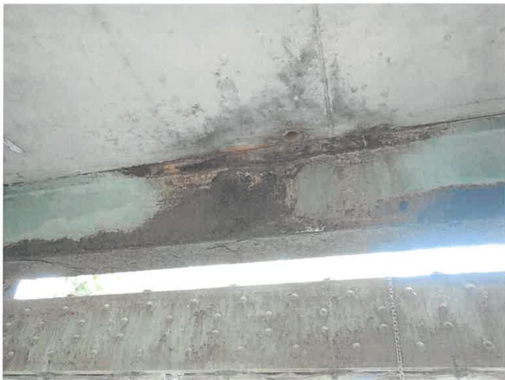
Photo 20: Stringer S1 east of Floorbeam FB2 with rust and section loss at midspan
