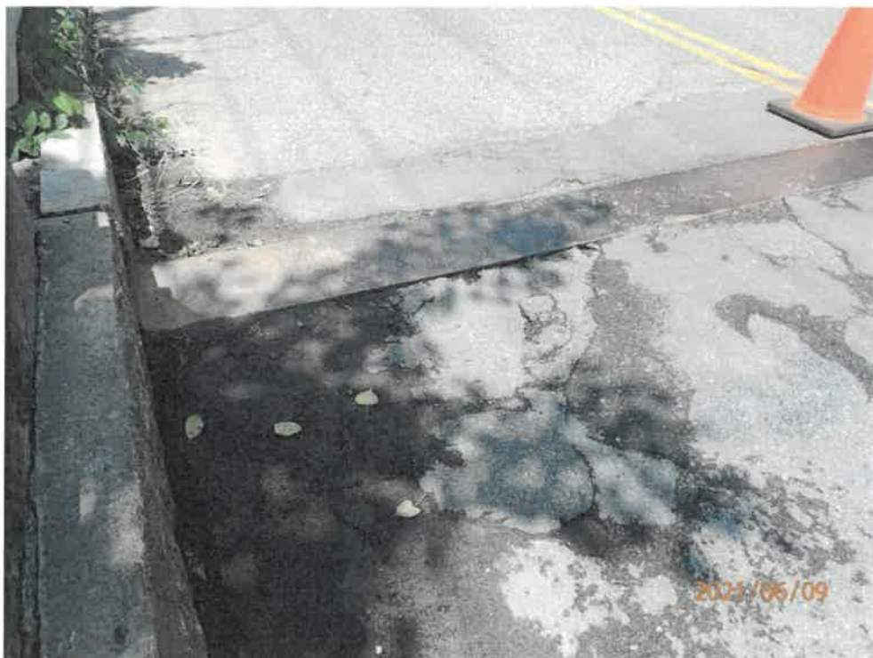
Photo 6: Eastbound Wearing Surface at the West Abutment deck joint, pothole with impacted sand and debris
