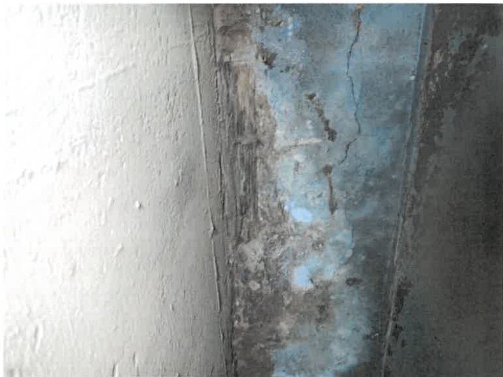
Photo 8: Underside of deck at the West Abutment between Stringer S2 and S3, spall with exposed rebar
