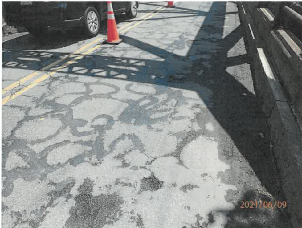
Photo 5: Eastbound travel lane wearing surface with sealed and unsealed cracks and potholes
