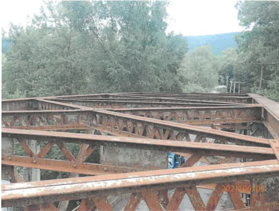
Photo 35: Upper Chord with typical rust and peeling paint
