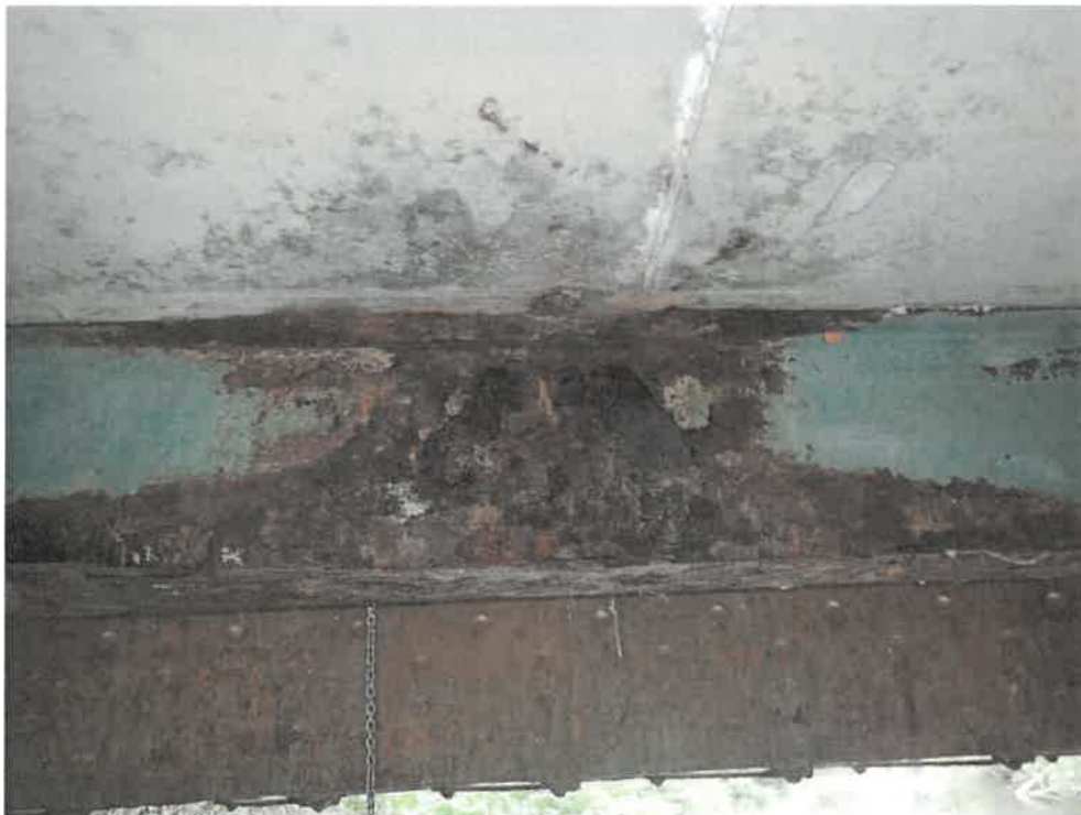
Photo 22: Stringer S5 between Floorbeams FB5 and FB6 with rust and section loss
