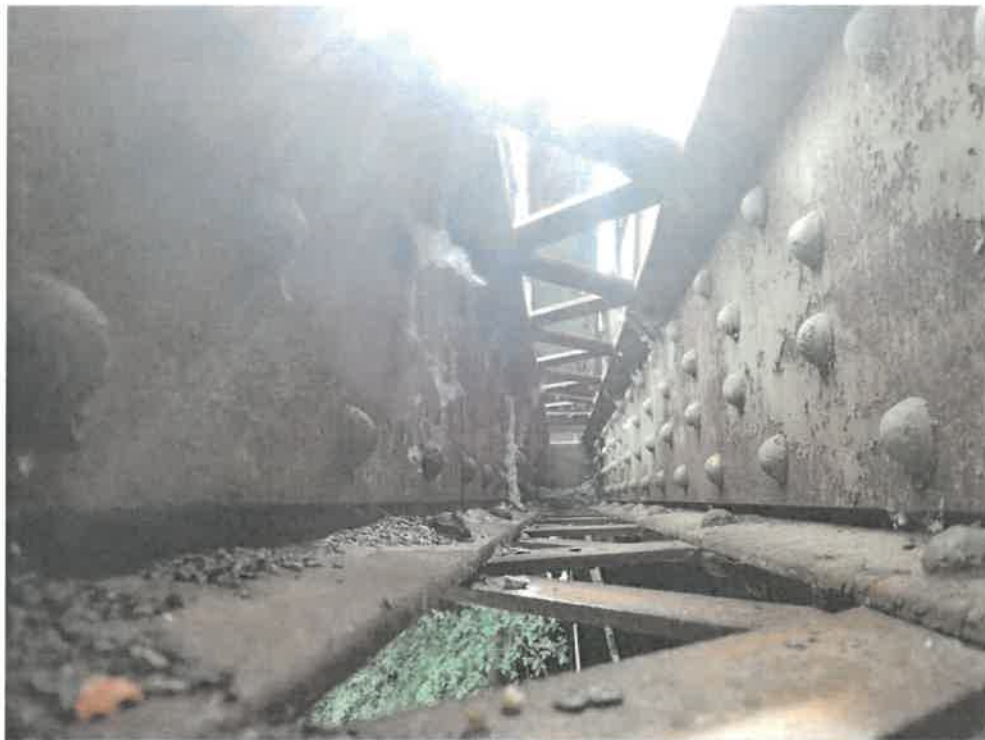
Photo 38: Lower Chord with typical rust and paint loss
