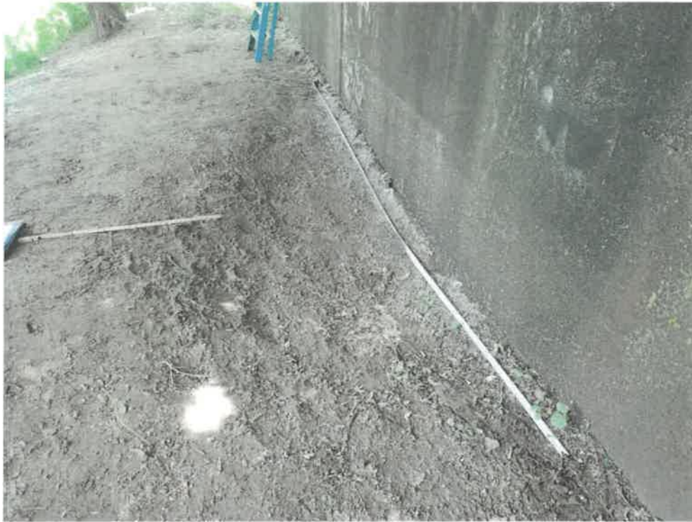
Photo 45: East Embankment, south end of East Abutment with depression
