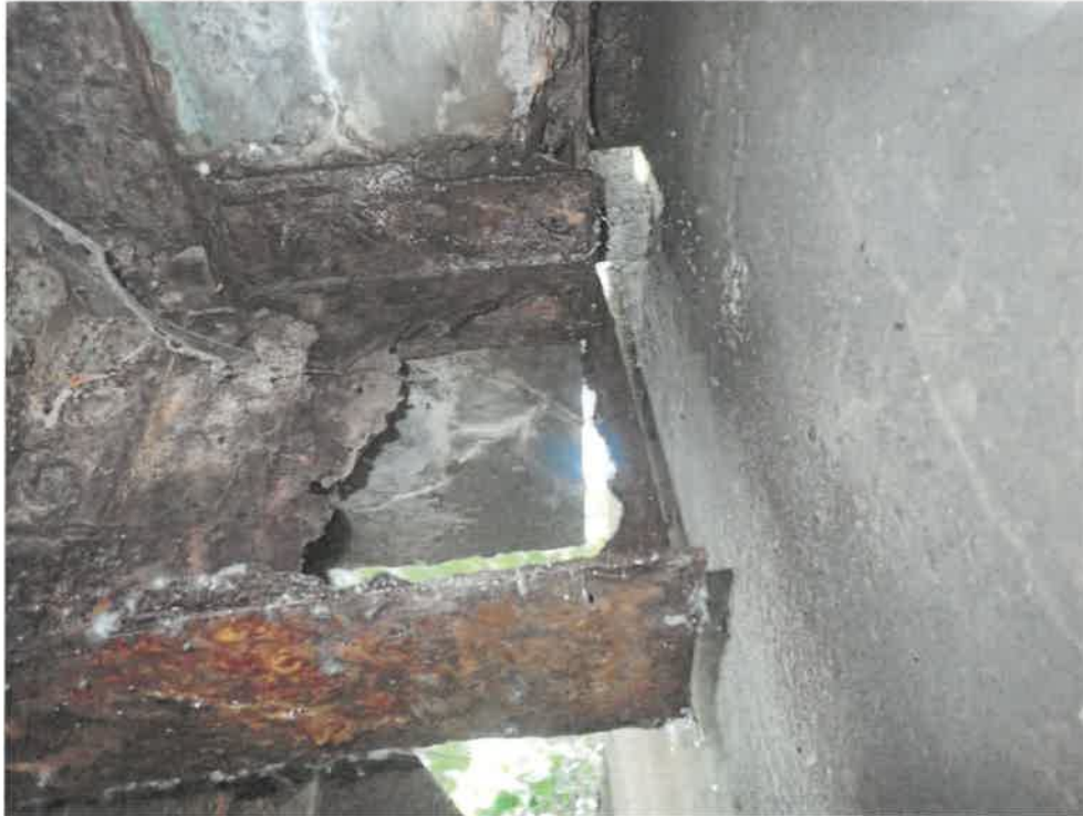
Photo 23: Stringer S1 at Floorbeam FB8 with perforation at end
