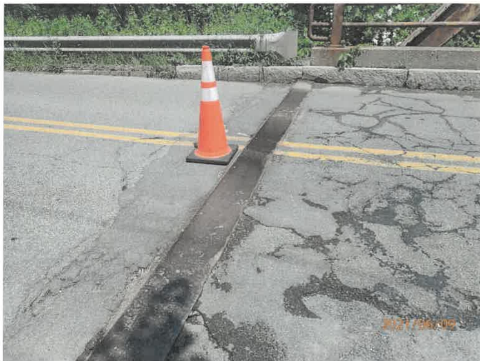
Photo 18: West Abutment deck joint; note potholes/spalls along the joint.
