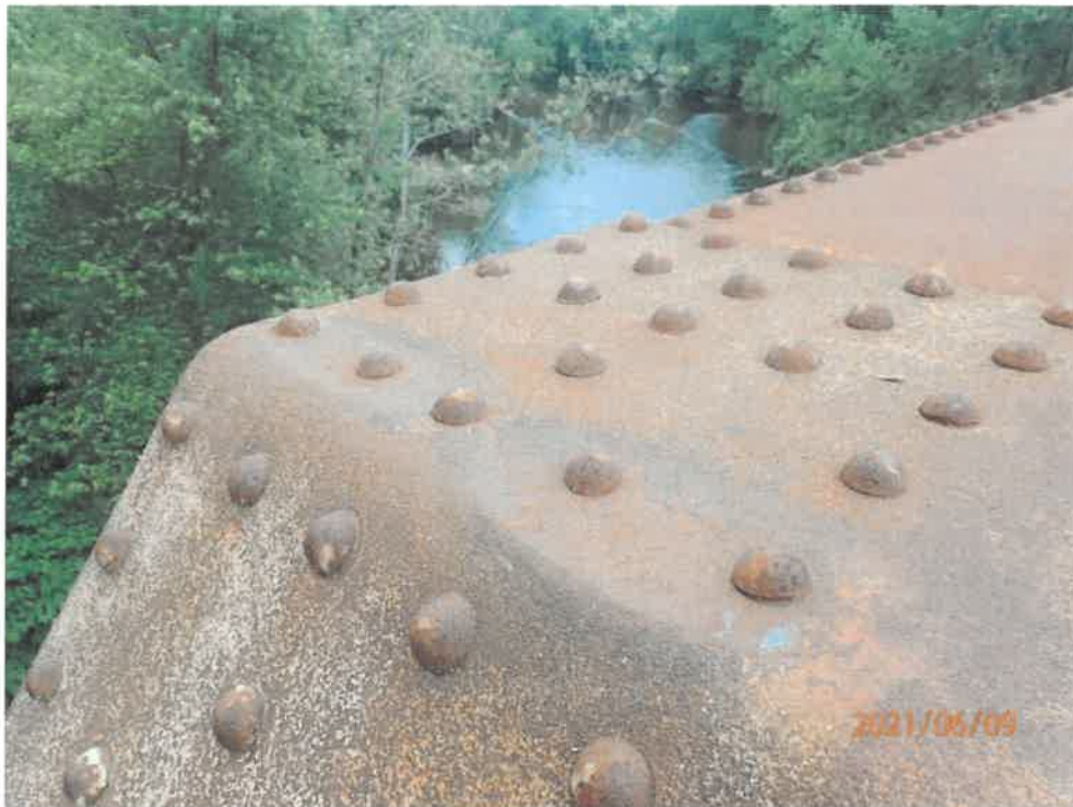
Photo 36: North Truss, U1 upper chord gusset plate with depressions/cupping
