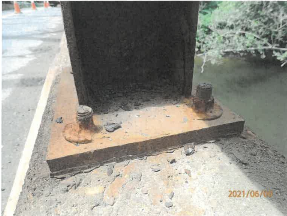
Photo 11: North Railing, 7th post from East Abutment, anchor bolt nuts with up to 100% section loss
