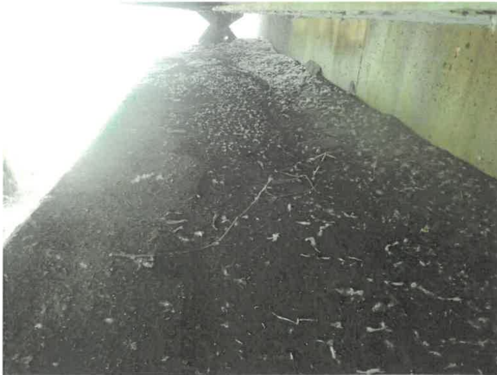
Photo 43: East Abutment bridge seat with debris accumulation
