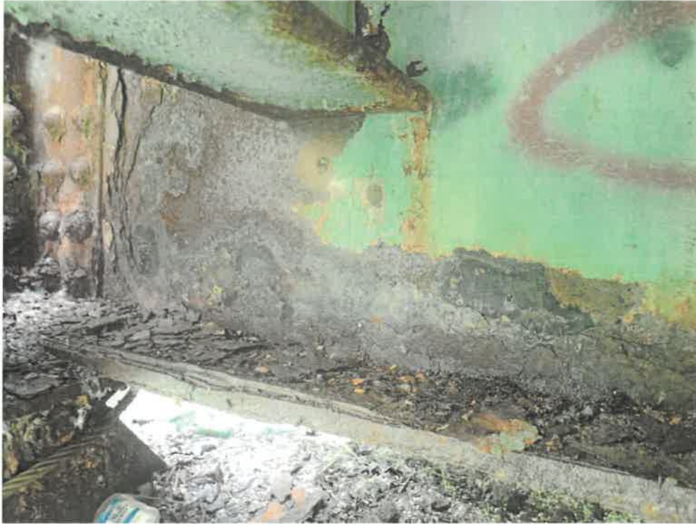
Photo 33: Floorbeam FB8 at north end, west face with heavy rust and section loss
