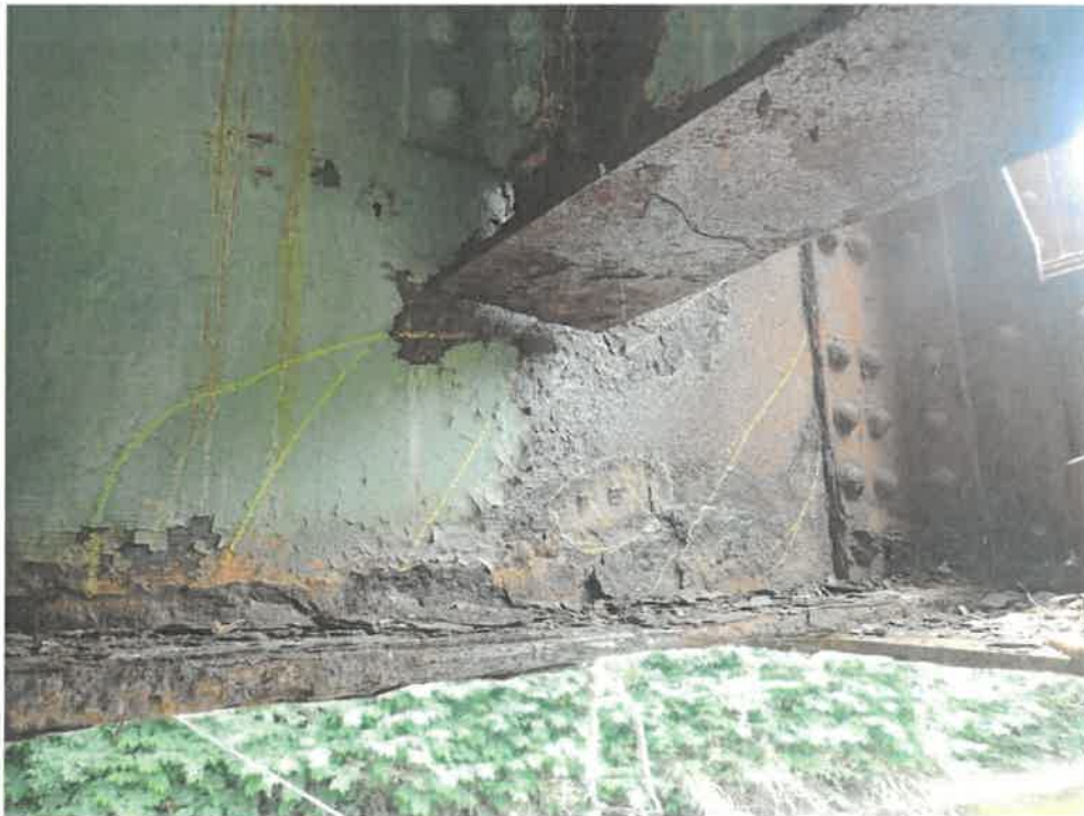
Photo 28: Floorbeam FB3 at south end, west face with heavy rust and section loss
