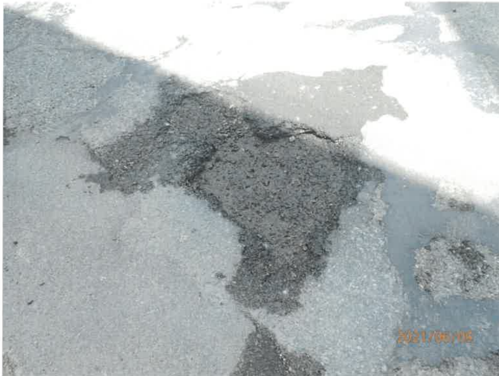
Photo 7: Eastbound Wearing Surface near the 13th rail post with a pothole
