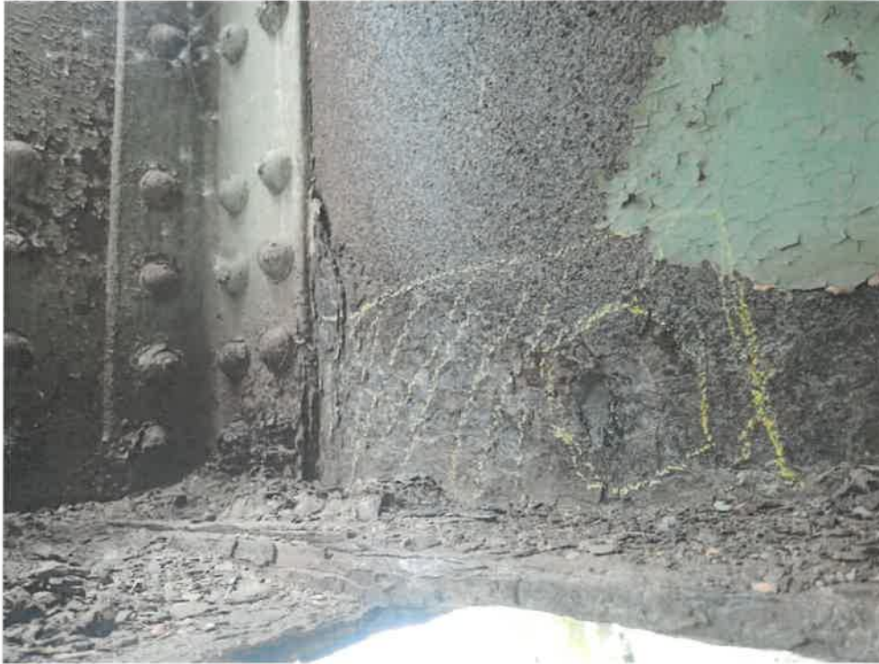
Photo 29: Floorbeam FB4 at north end, east face with heavy rust and section loss
