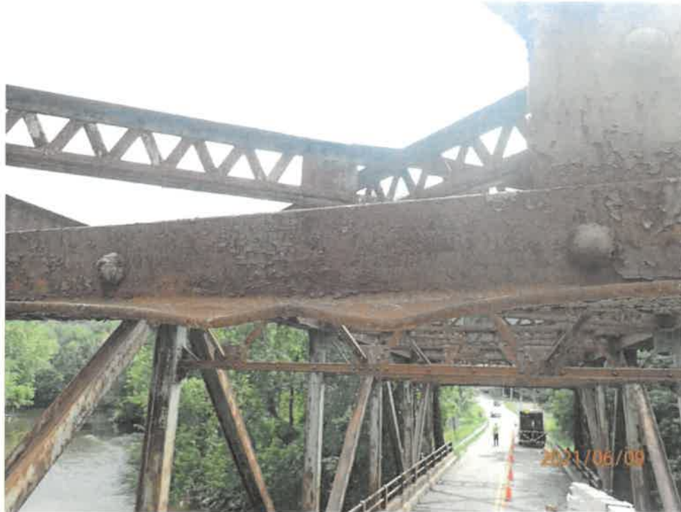
Photo 39: U2 Sway Bracing with collision damage
