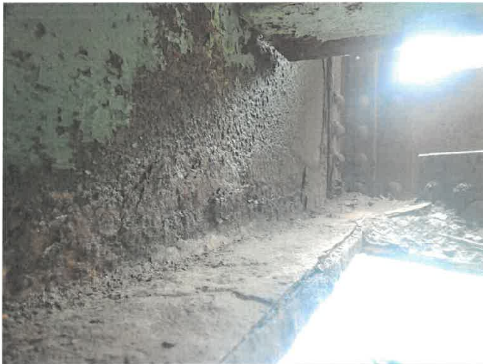
Photo 26: Floorbeam FB1 at south end, west face with heavy rust and section loss
