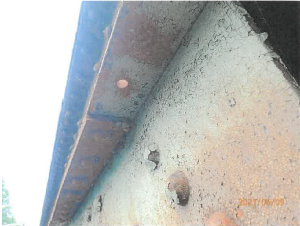
Photo 37: South Truss, U3 south face with missing rivet at upper chord
