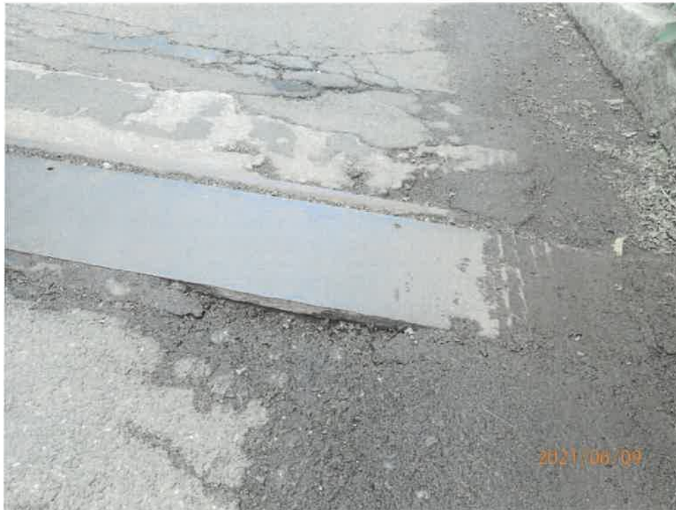
Photo 17: East Abutment deck joint spall exposing joint armor edge and approach pavement cracked with some break-up
