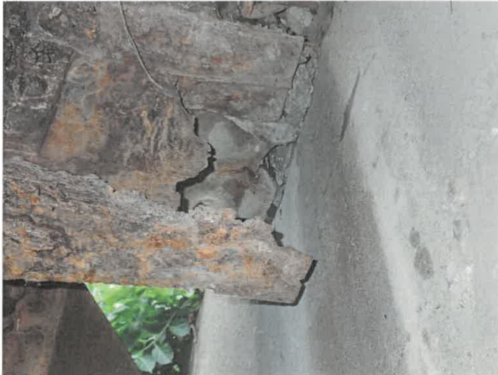
Photo 19: Stringer S5 at Floorbeam FB0 (west end) with rust perforation at end
