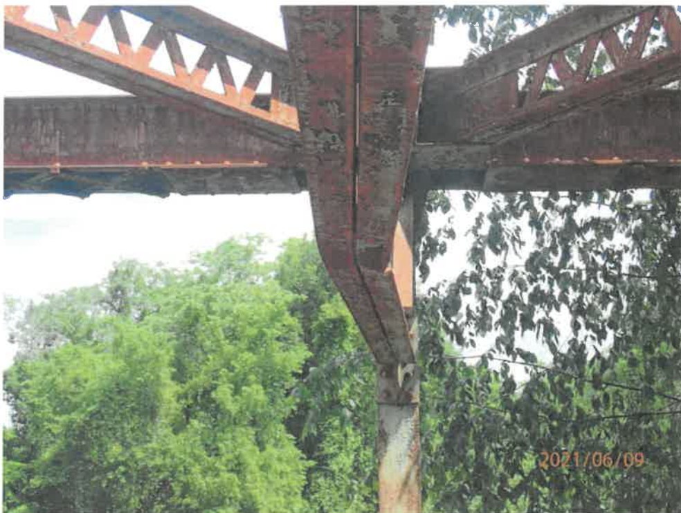
Photo 40: U6 Sway Bracing with collision damage
