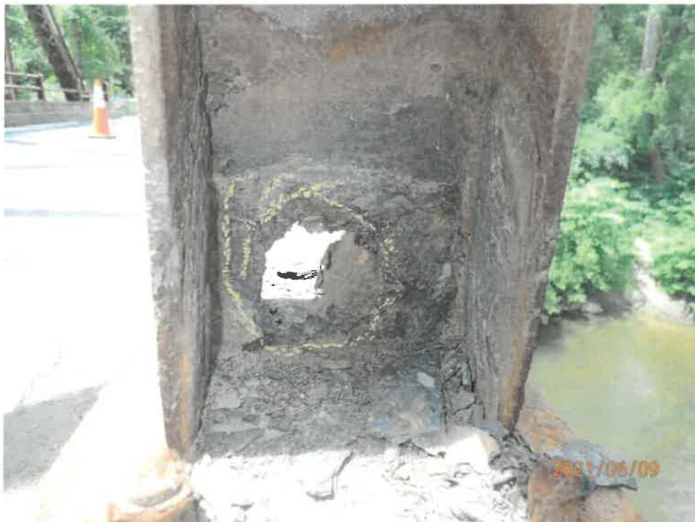
Photo 12: North Railing, 11th post from East Abutment with perforation in lower web
