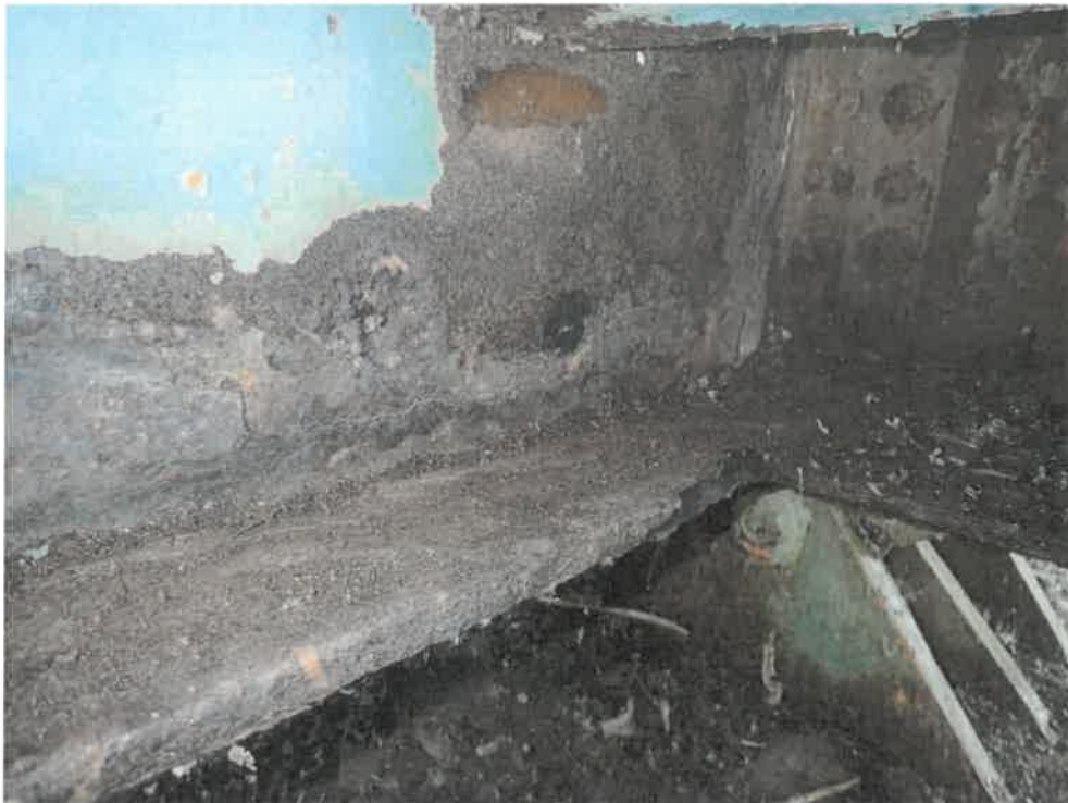
Photo 34: Floorbeam FB8 at south end, west face with heavy rust and section loss
