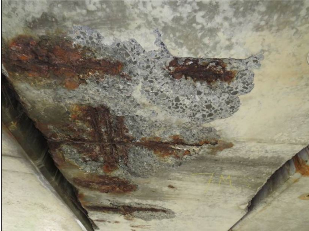
P-10-002 (0DY) SPALLING AND EXPOSED TENDONS (BEAM 7)
