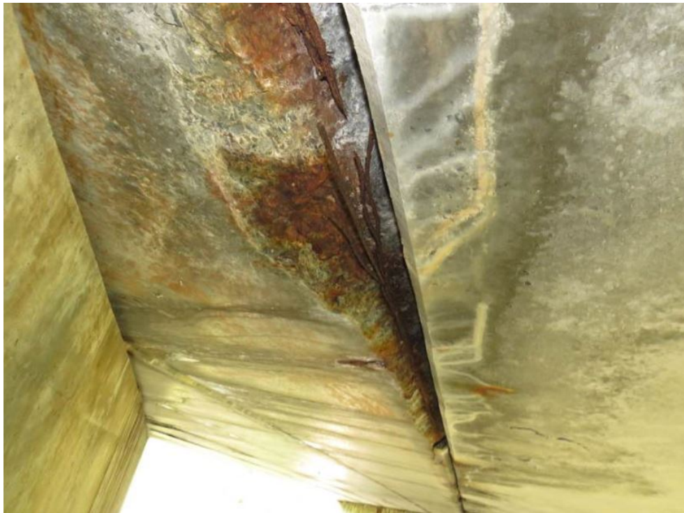
P-10-002 (0DY) SPALLING AND EXPOSED TENDONS (BEAM 6)
