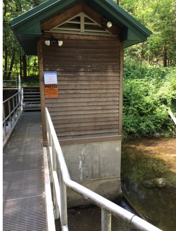
Karner Brook Raw water Pump Station
