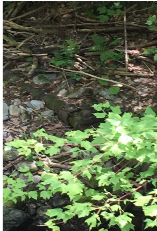
Old Karner Brook transmission Main and Shut-off Valve
