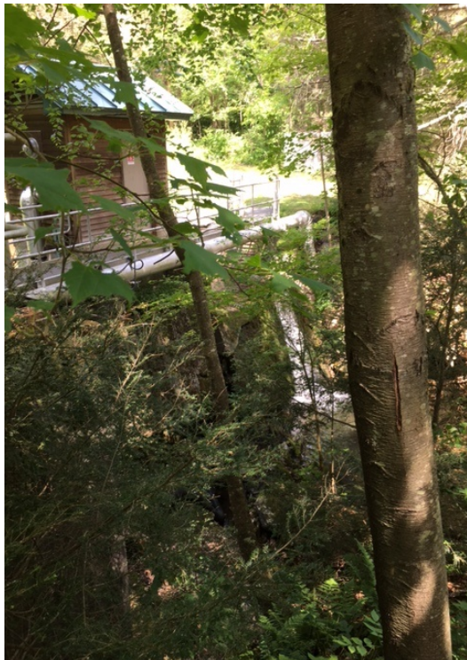
Karner Brook Reservoir Dam- Unsafe
