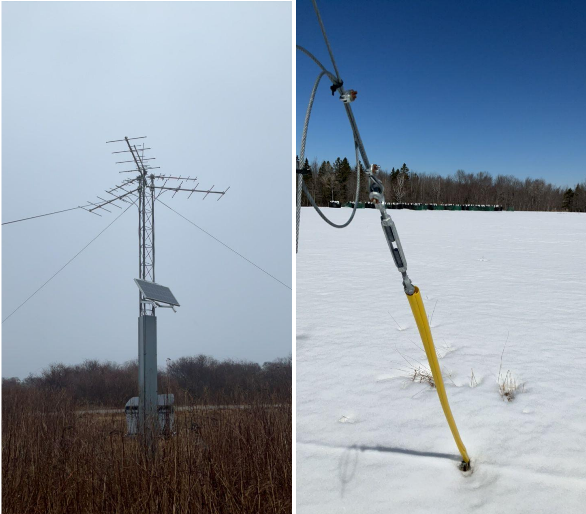
Figure 3: Anti-climb panels and marked guy line on Motus receiver station similar to proposed installation.
