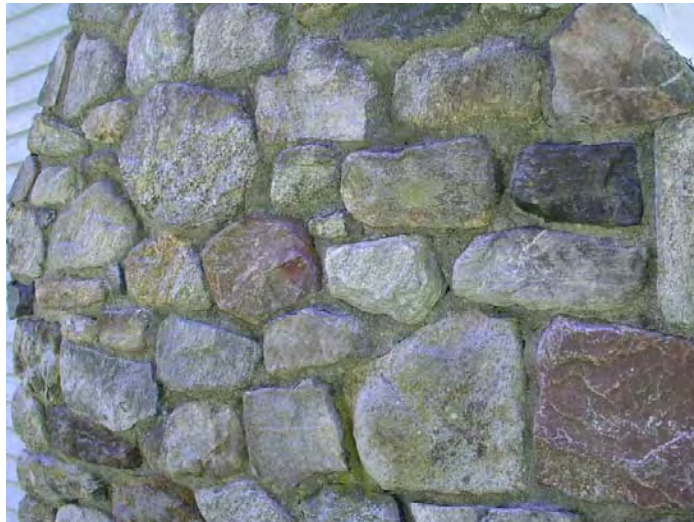
Fig. 5.9. Stone masonry needs spot-repointing.
