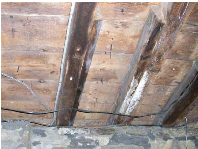
Fig. 6.10. First floor framing evidencing mold growth.
