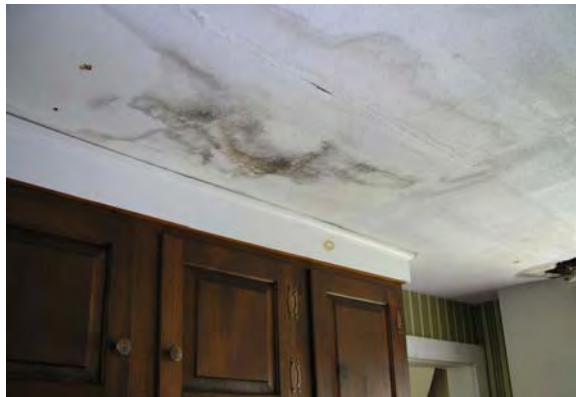
Fig. 6.5. Water damage and mold at kitchen ceiling.
