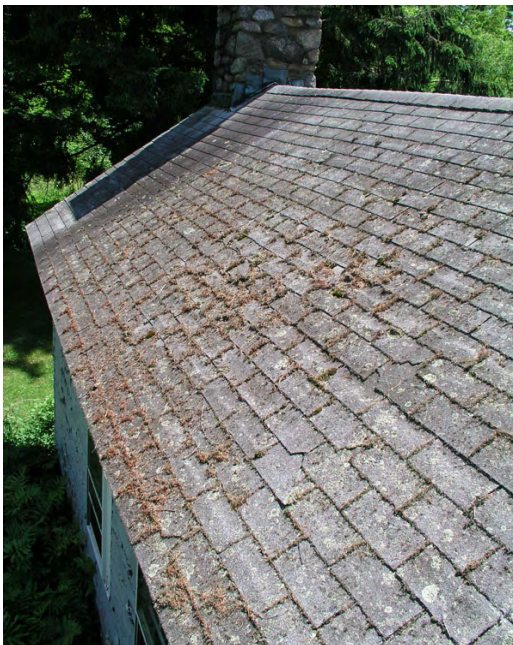
Fig. 5.2. Condition of shingles at ell.
