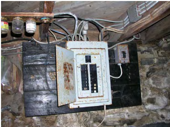
Fig. 4.4. Main distribution panel.
