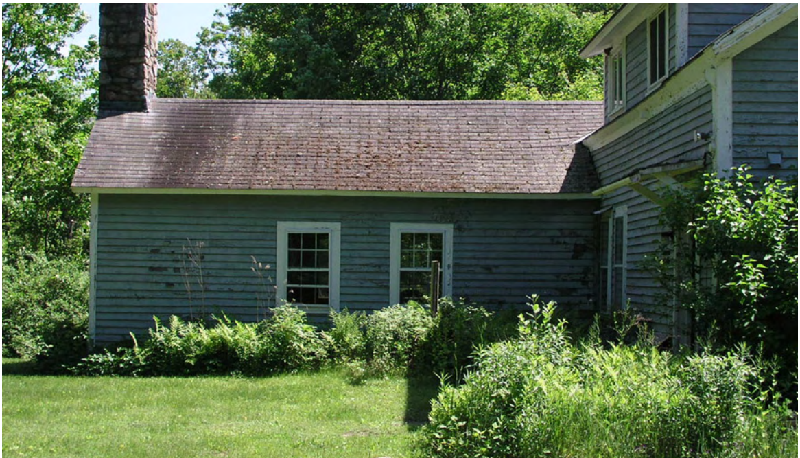
Fig. 1.5. Landscaping and “mulched-up” grade adjacent to house. As part of a coordinated effort to re-route roof drainage, the grounds should be regraded to pitch away from the building.
