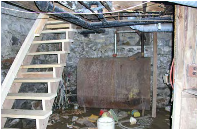
Fig. 4.5. Existing 275-gallon oil tank.
