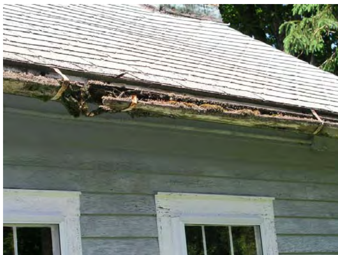
Fig. 5.4 Rotted gutter section.
