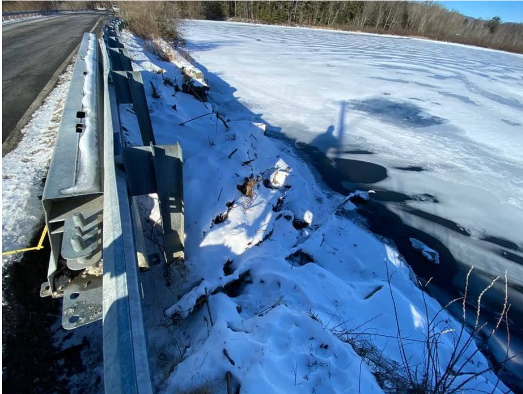
Photo 3: Debris blocking the north end of the pipe and the collapsed north headwall.
