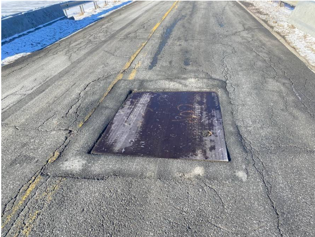
Photo 6: Cracking and plate in the wearing surface.
