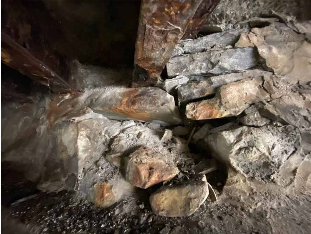
Photo 13: Area of missing and loose stones in the south breastwall under beams 3 & 4.
