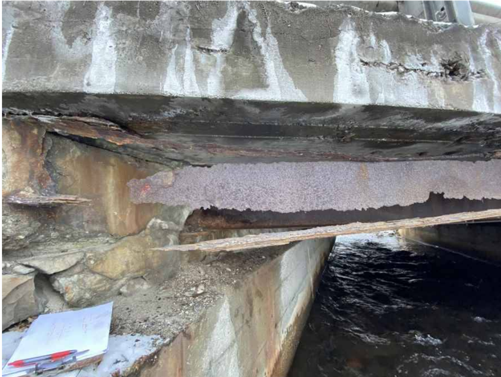
Photo 11: East elevation, beam 19 failed. Note, out of service.
