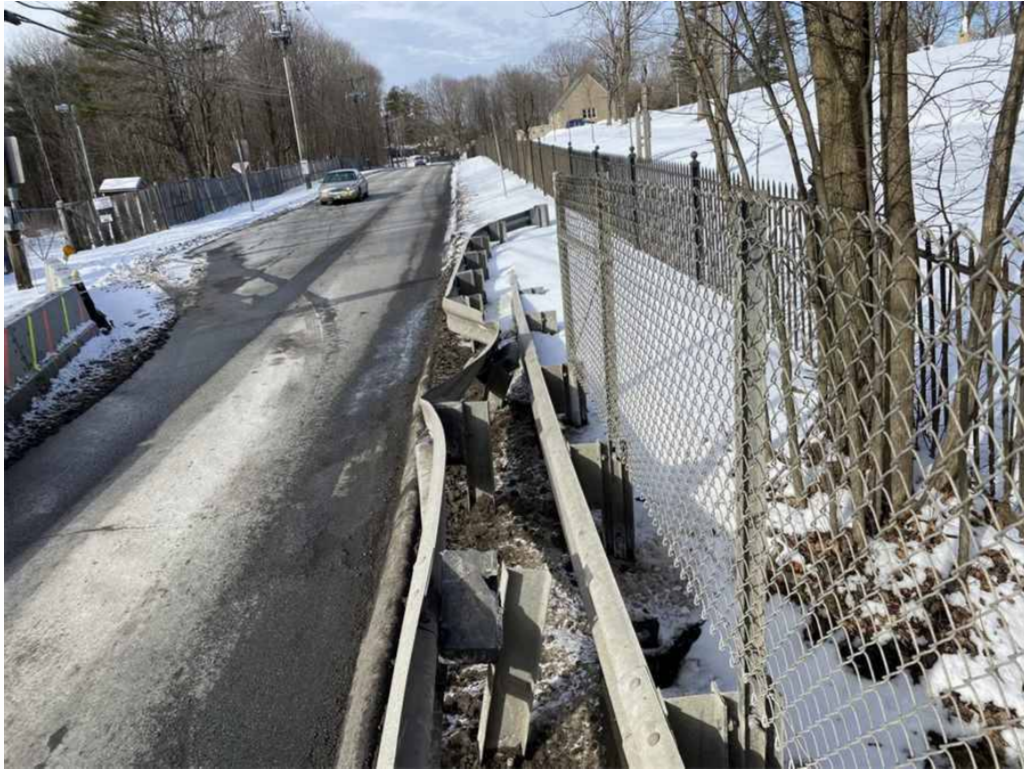
Photo 5: East bridge guardrail with tear and impact damage.
