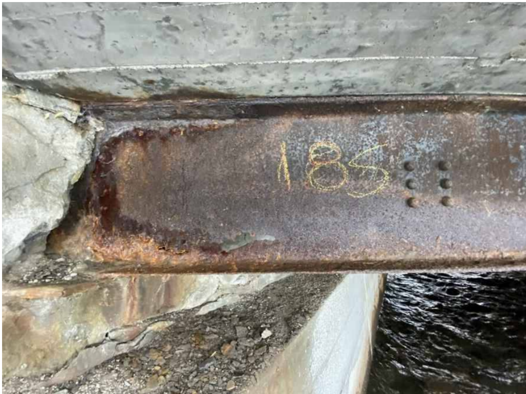
Photo 10: Beam 18, south end, with section loss and holes.
