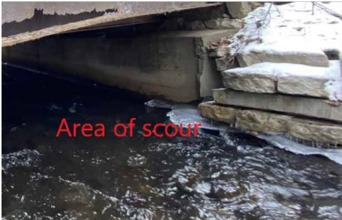
Photo 14: North curtain wall scour.
