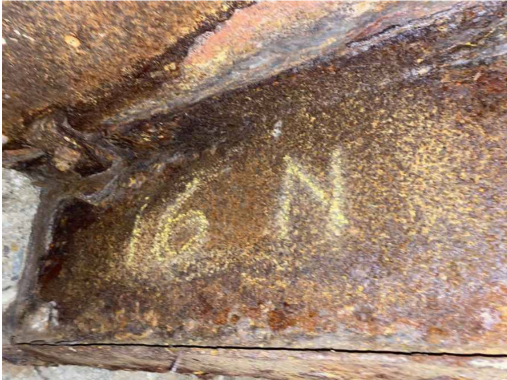
Photo 9: Beam 16, north end, with section loss.
