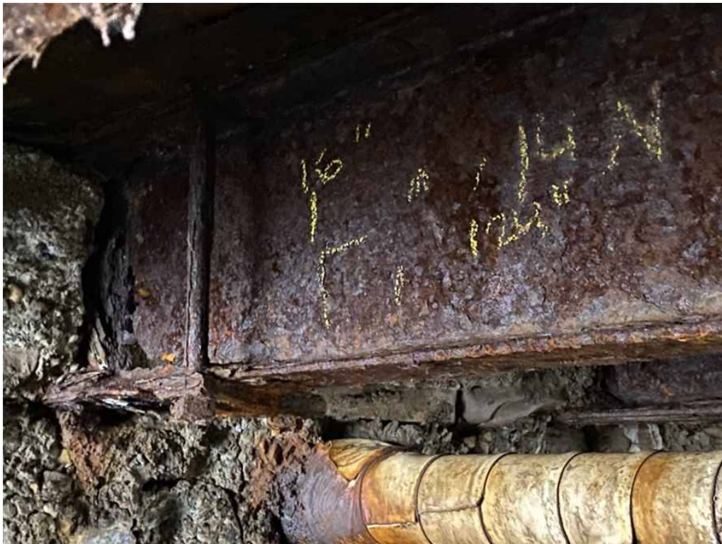
Photo 8: Beam 14, north end, with section loss and holes.
