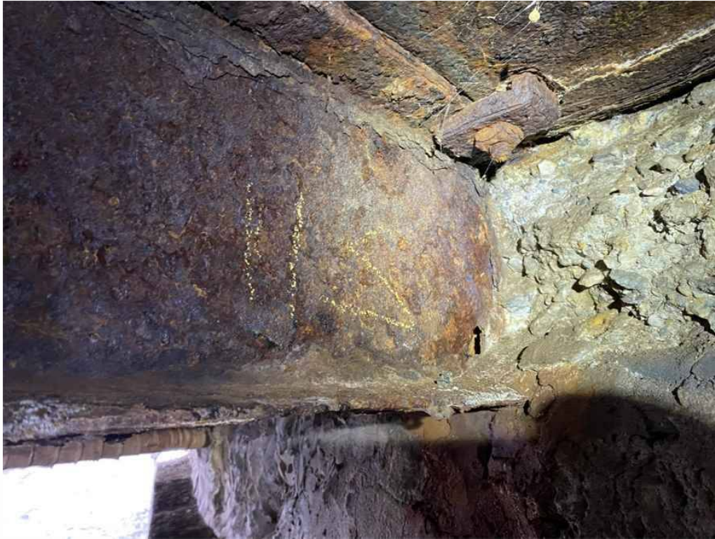
Photo 7: Beam 11, south end, with section loss and holes. Note, out of service.
