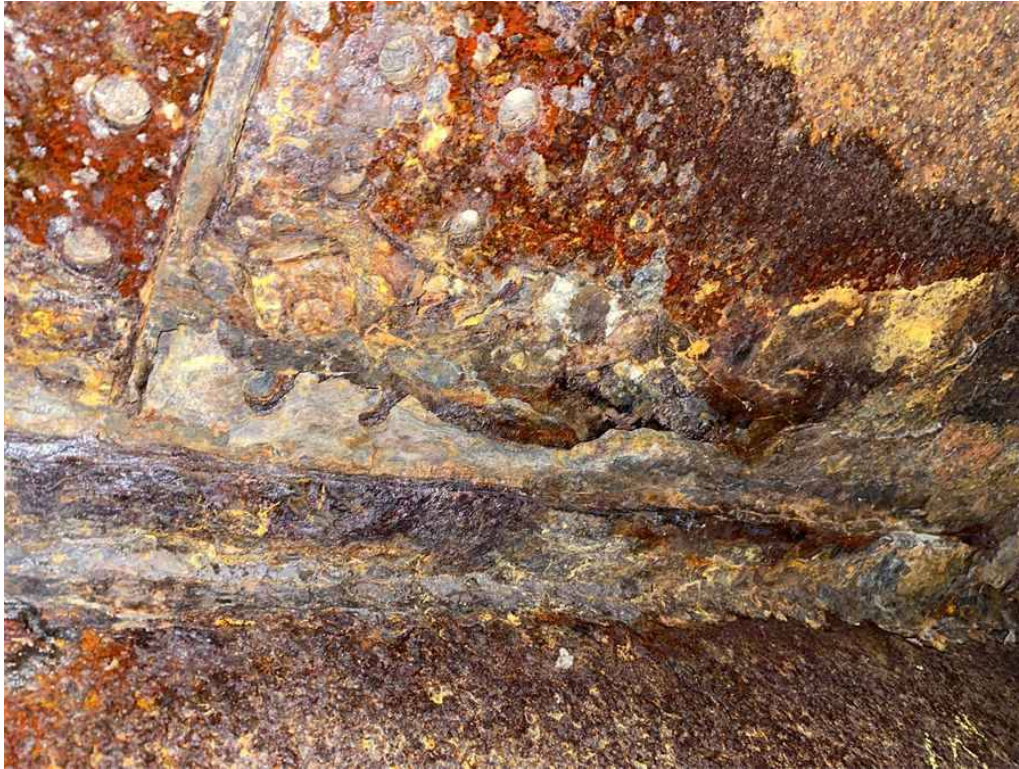
Photo 3: Typical stay in place form condition, with section loss and holes. Note the concrete behind the steel plate.
