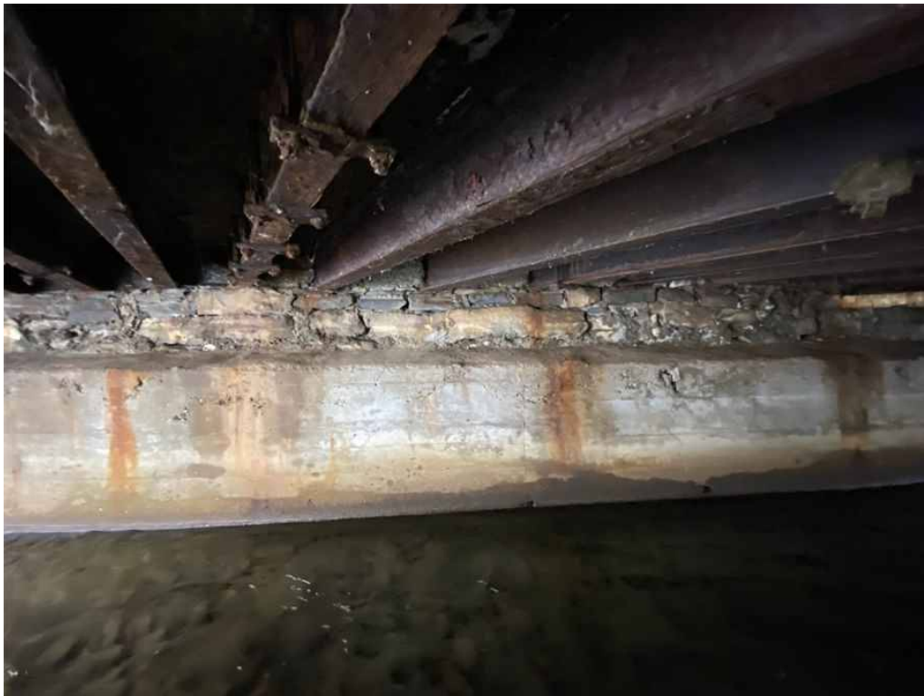
Photo 12: North breastwall condition.
