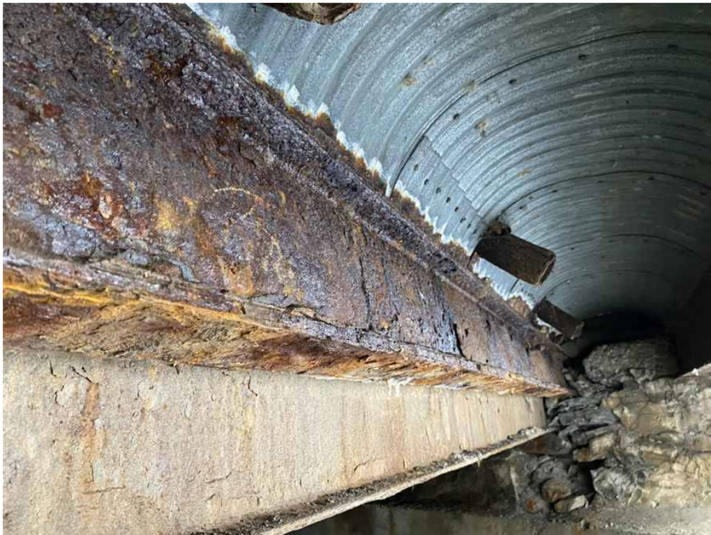
Photo 4: Bay 2, looking south, jack arch and drain pipe condition. Also, note the beam 3 rusting and section loss.
