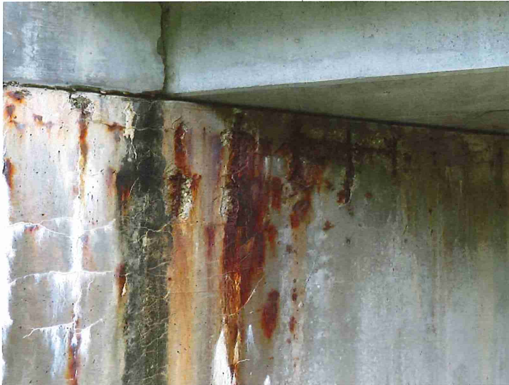
Photo 11: Spalls, cracking and rust staining at the south end of the west breastwall.
