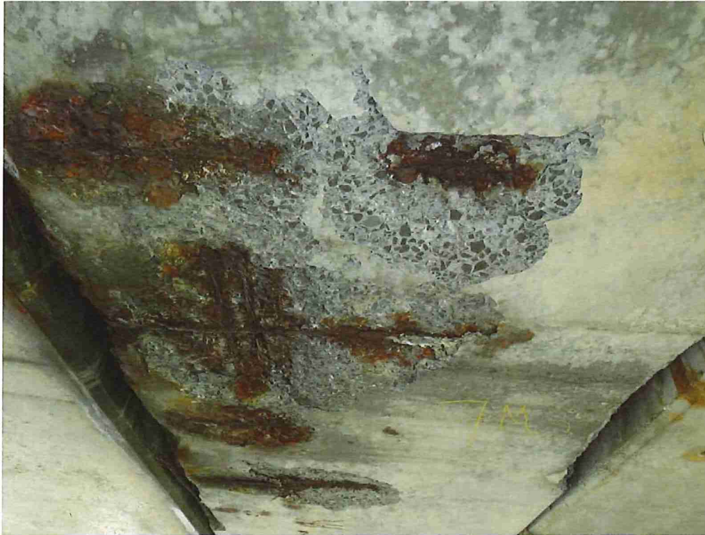
Photo 7: Beam 7 at 40' from the west abutment. Note all of the exposed tendons.
