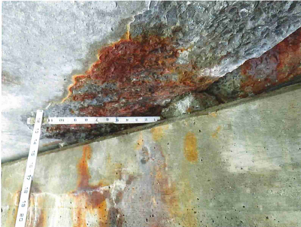
Photo 5: Spall at the west end of beam 7 with one exposed tendon.
