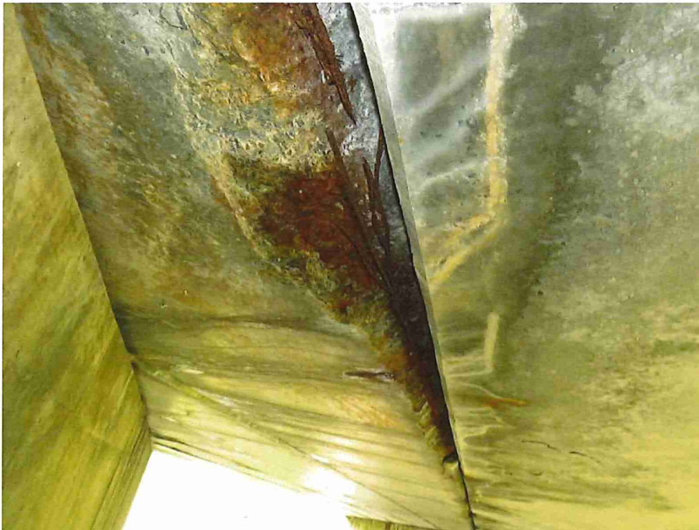
Photo 8: Spall and severed tendon at the west end of beam 6.
