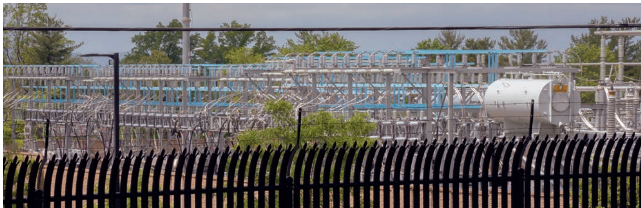
New energy substations are often constructed near data centers to help lower the voltage to the rates the facilities need. (Dave Harp)
