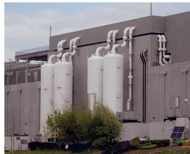
Chilled water storage tanks appear on the side of a data center in Loudoun County, VA. Such systems are for backup cooling, according to the company's website. (Dave Harp)
