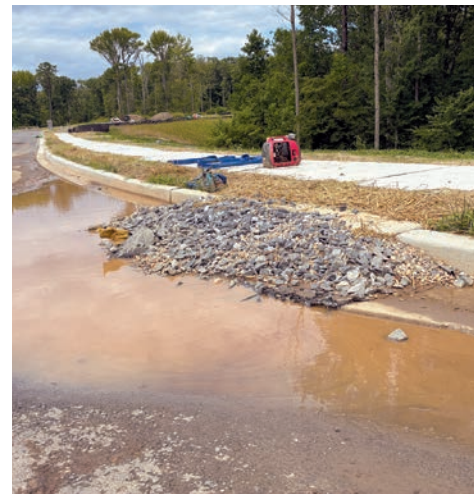
Muddy water stands in a yet unbuilt section of the Ridgely's Reserve housing development in Harford County, MD. (Timothy B. Wheeler)
