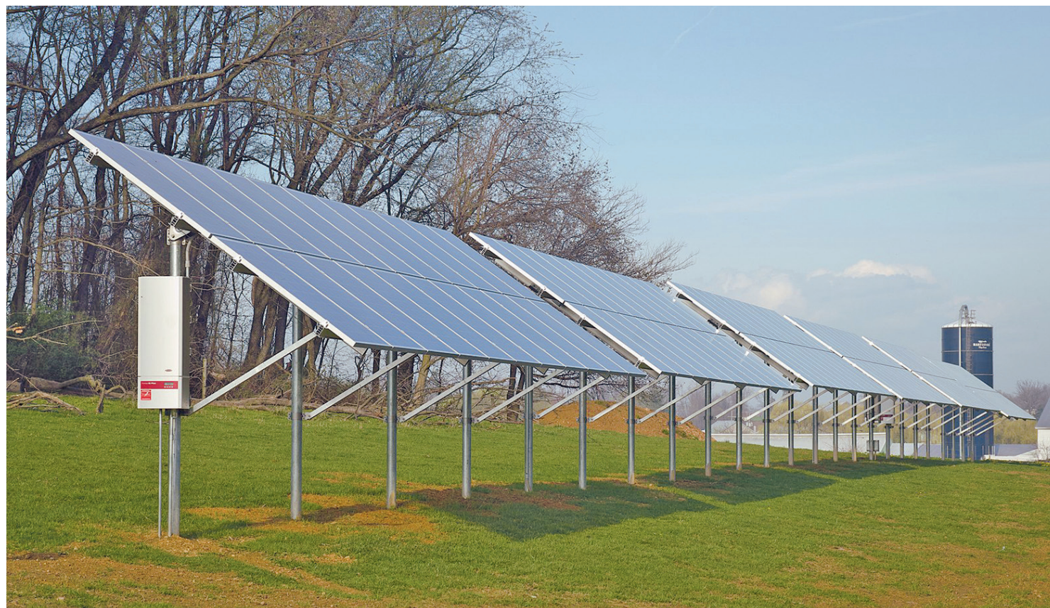
These solar panels, shown here in 2011, were installed as part of a 240-panel array at Seldom Rest Farms in Myerstown, PA, to generate energy for the farm, as well as for a neighboring farm and homes on the local electrical grid. (U.S. Department of Agriculture)
