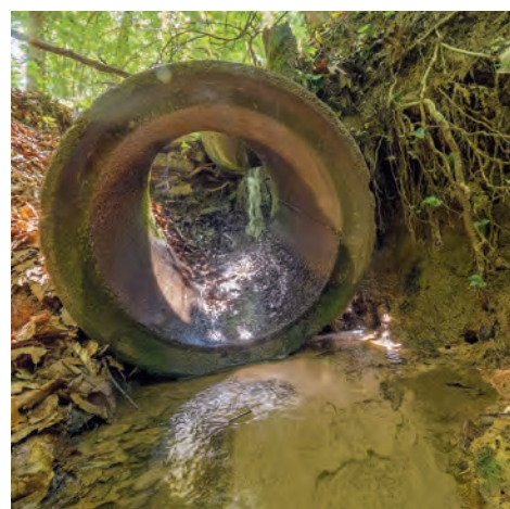
A broken pipe rests at the lower end of a buried stream in DC’s Fort Dupont Park. (Dave Harp)
