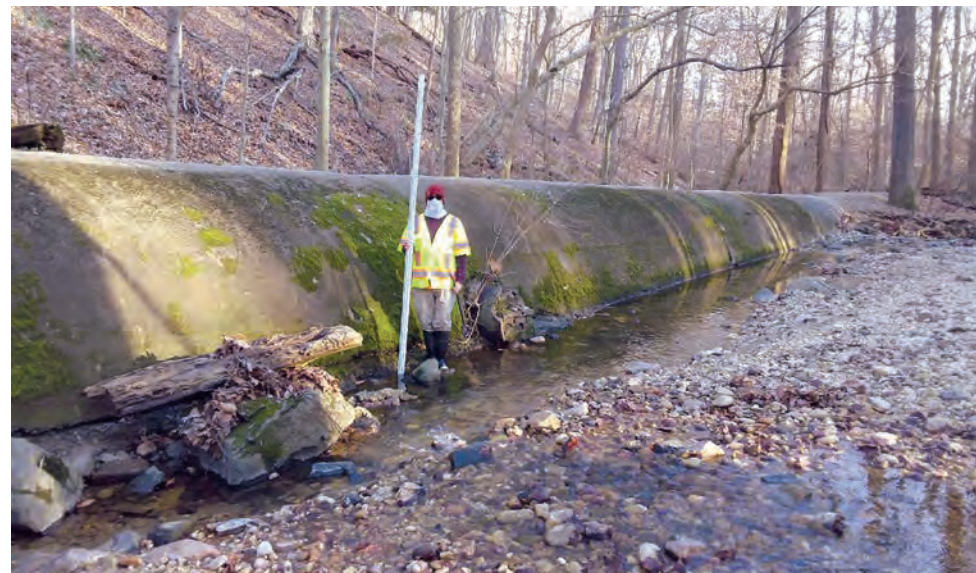
This large pipe carries a portion of Foundry Branch through the District of Columbia. (Straughan Environmental)
