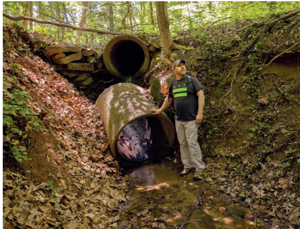
Josh Burch, an environmental protection specialist with the District of Columbia's Department of Energy and Environment, inspects a section of pipe that carries a buried stream through Fort Dupont Park, just east of the Anacostia River. The stream is slated to be "daylighted," or brought to the surface, to restore its ecosystem functions to the landscape. (Dave Harp)
