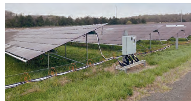
The Remington Solar Power Facility on 125 acres in Fauquier County, VA, was developed as a public-private partnership between the state and Microsoft. (Meg Cole)
