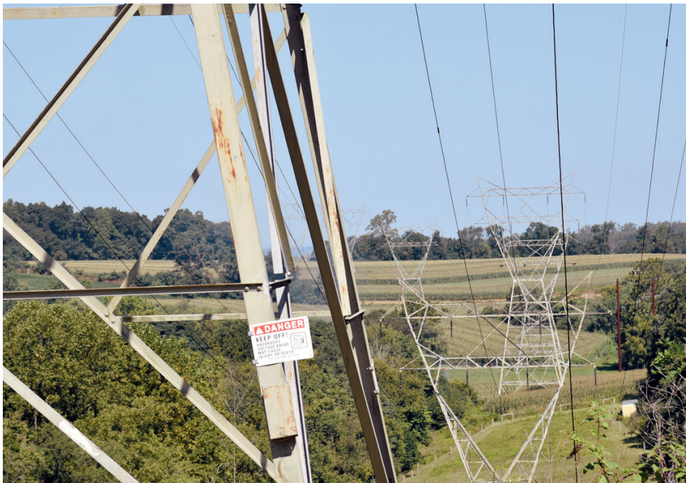
High-voltage transmission lines march through farmland in Lancaster County, PA. (Ad Crable)
