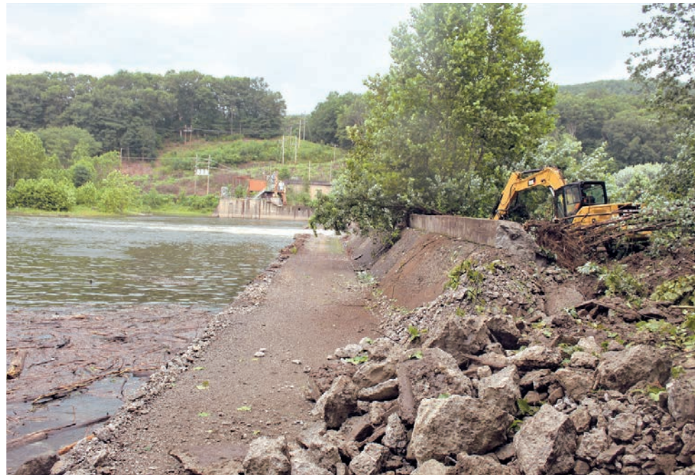
The Oakland Dam is removed from the North Branch of the Susquehanna River in Pennsylvania. (Courtesy of Endless Mountains Heritage Region)
