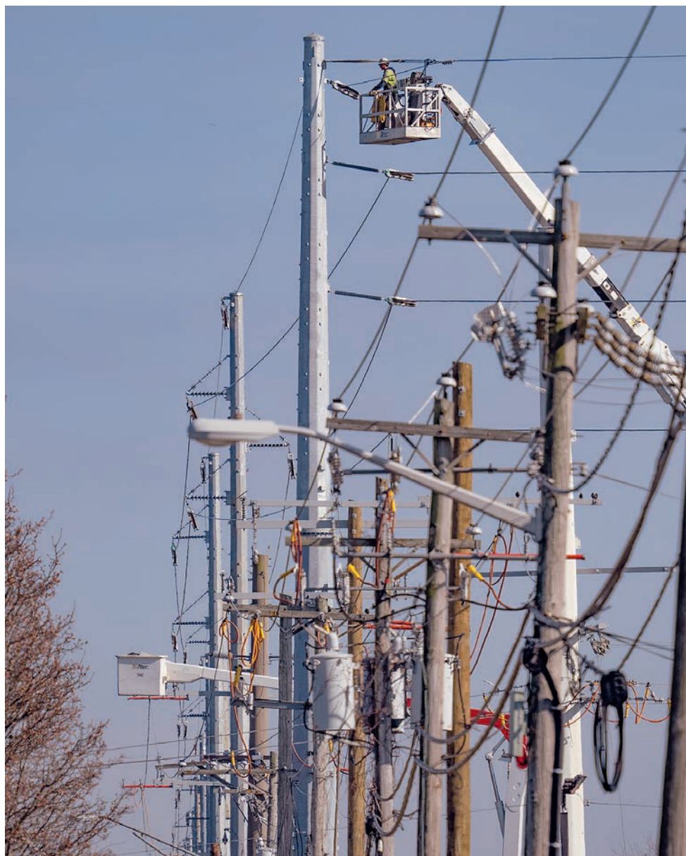
A technician works on a power grid update along Route 50 in Cambridge, MD. (Dave Harp)
