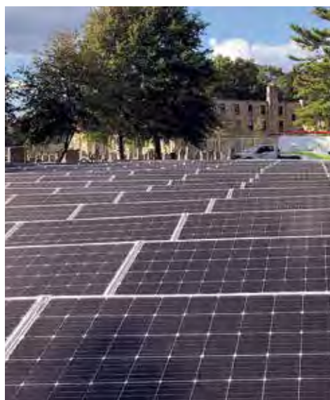
The Monastery of Our Lady of Mt. Carmel in northeastern DC allowed this community solar project to be built on its property. It saves about 50 local families $500 a year on their electric bills. (Ipsun Solar)
