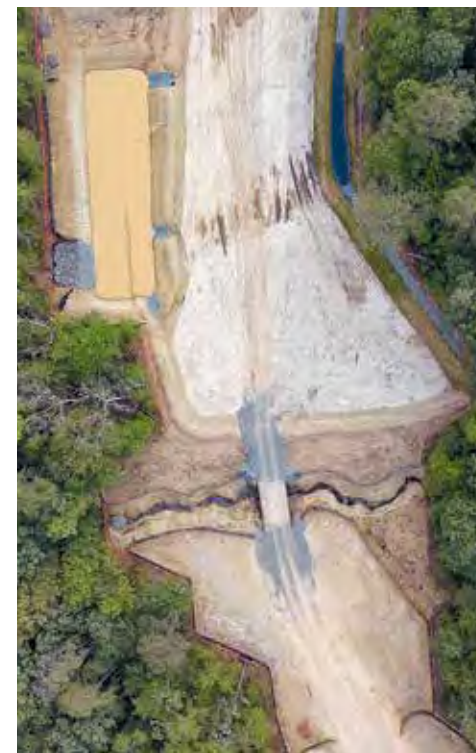
A sediment pond collects runoff near a passage through the forested construction site in Harford County, MD. (Nick Chryst)
