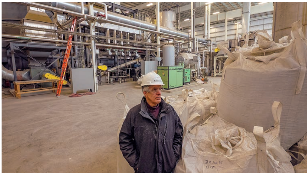
Pat Thompson leads a tour of the EnergyWorks plant in Gettysburg, PA, in 2015 during one of the few times it was operating after construction was completed in 2013. (Dave Harp)
