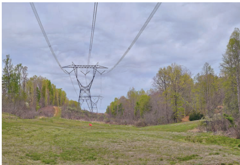
A 765-kilovolt transmission line passes by the backyard of a private home before connecting to the Joshua Falls substation near Lynchburg, VA. (Lauren Hines-Acosta)
