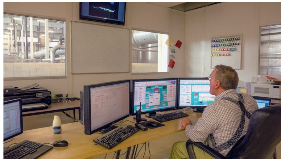
At EnergyWorks, the process of treating poultry manure to remove nutrients and generate electricity can be guided by two people mostly working in a control room. (Dave Harp)
