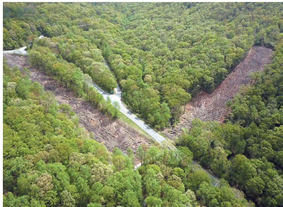
Brown swaths in this 2018 photo mark the areas where trees were cut near Charlottesville, VA, to make way for the Atlantic Coast Pipeline, but the project has been cancelled. (Curtis Sheets)
