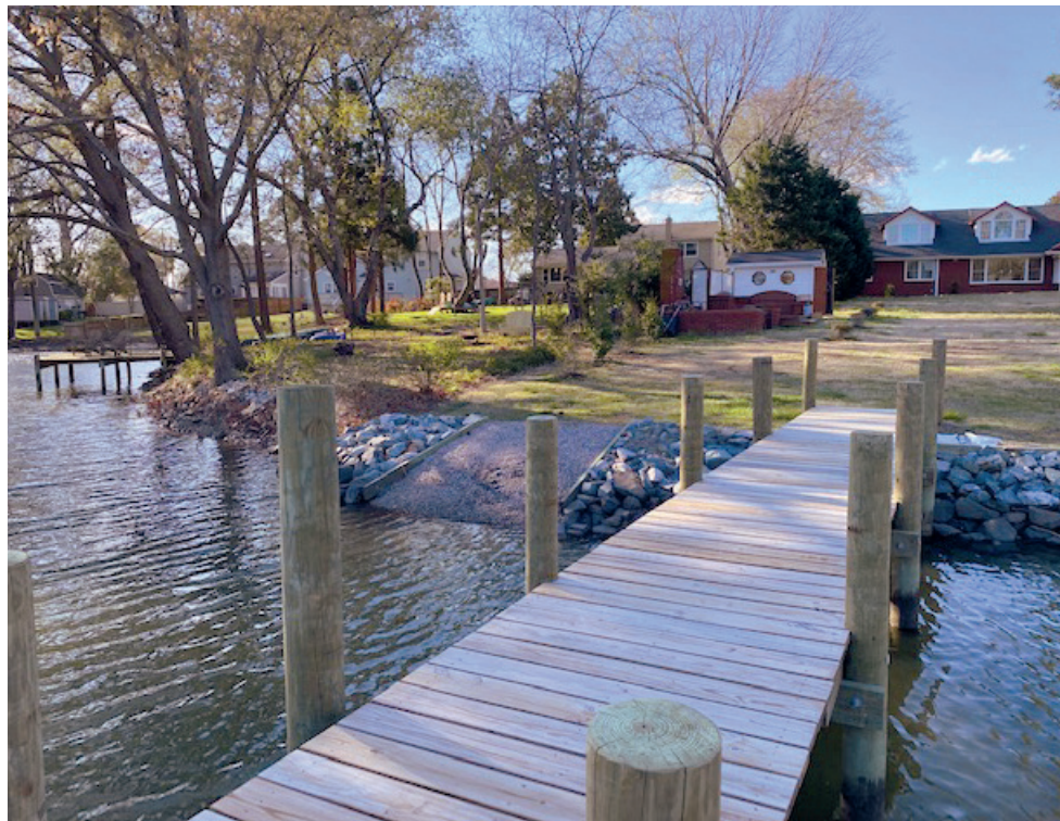
A contractor who built a permitted pier along this shoreline in Hampton Roads, VA, added stone and a gravel kayak ramp without getting a necessary permit required under the state's living shorelines law. The landowners tried to correct the issue by adding living shoreline elements but were denied a permit three times. (Courtesy of Mary Swift)
