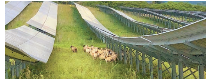
Sheep graze between and under solar panels that help power Susquehanna University in Pennsylvania. (Owens Farm)
