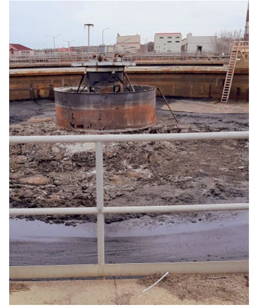
Solids are built up in an inactive settling tank at Baltimore's Back River Wastewater Treatment Plant during a state inspection of the facility on March 22, 2022. (Courtesy of Maryland Department of the Environment)
