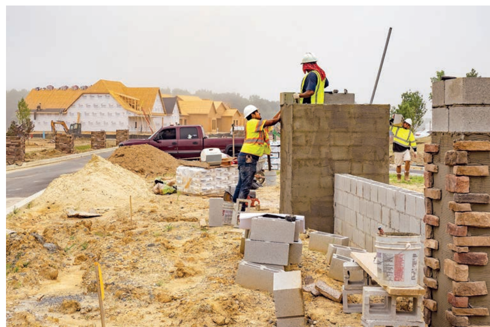
Masonry workers build an entrance at the Lakeside development in Trappe, MD. (Dave Harp)
