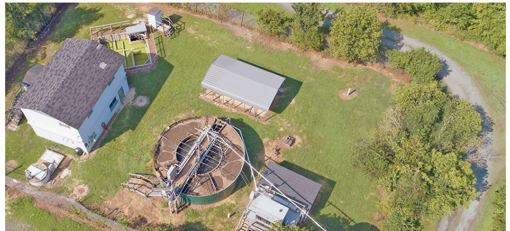
This mobile home community wastewater treatment plant along Sands Road in Anne Arundel County, MD, is among five such plants that have been in repeated noncompliance in recent years. No enforcement action has been taken. (Dave Harp)
