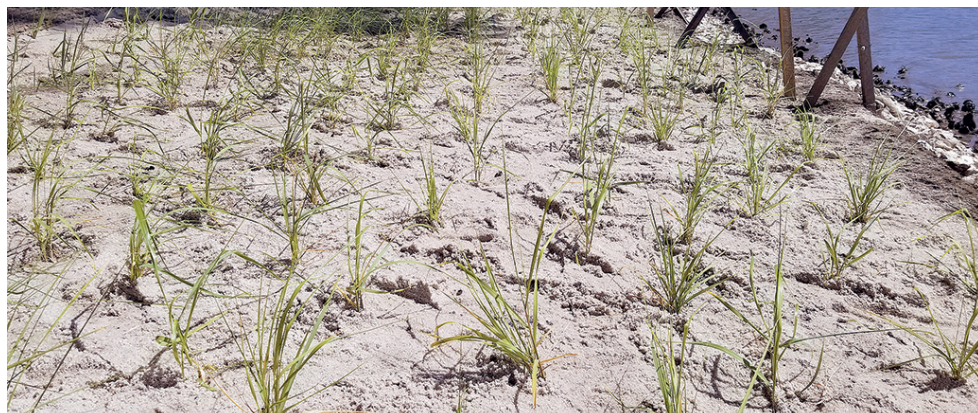
Plugs of grasses are planted in sand as part of a living shoreline project on private property along Virginia's Elizabeth River. Rather than hardening the shore's edge with concrete or riprap, living shorelines create natural edges that receive the water's ebb and flow and, over time, can be more resilient in the face of rising sea levels and powerful storms. (Sterling Rollings)
