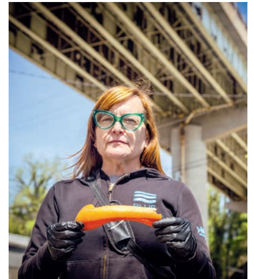
Leanna Frick of Blue Water Baltimore holds a large patch of lead-tainted paint that fell from the 28th Street bridge behind her. (Courtesy of Blue Water Baltimore)
