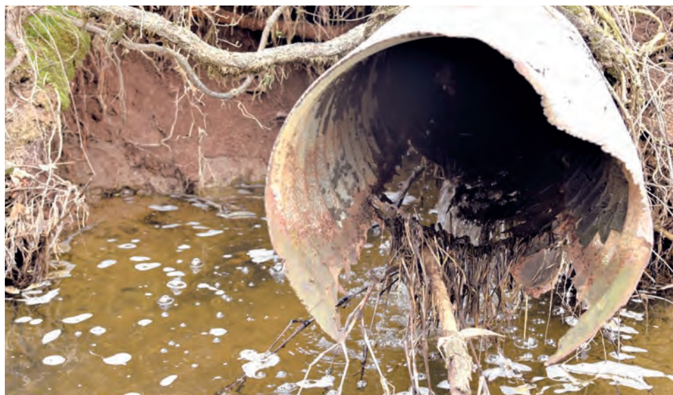
This rusting discharge pipe is causing erosion and threatening a dike that forms wetlands in Pennsylvania’s Middle Creek Wildlife Management Area. (Ad Crable)
