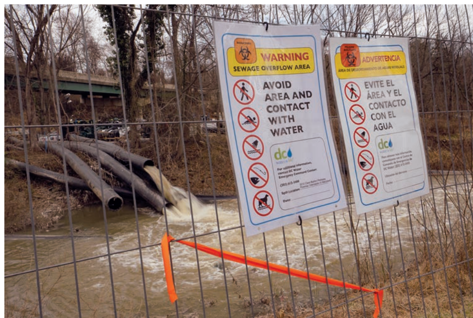
Raw sewage from the January 2026 pipe collapse near the District of Columbia was diverted into the C&O Canal, then pumped back into the sewer line farther downstream. (Dave Harp)
