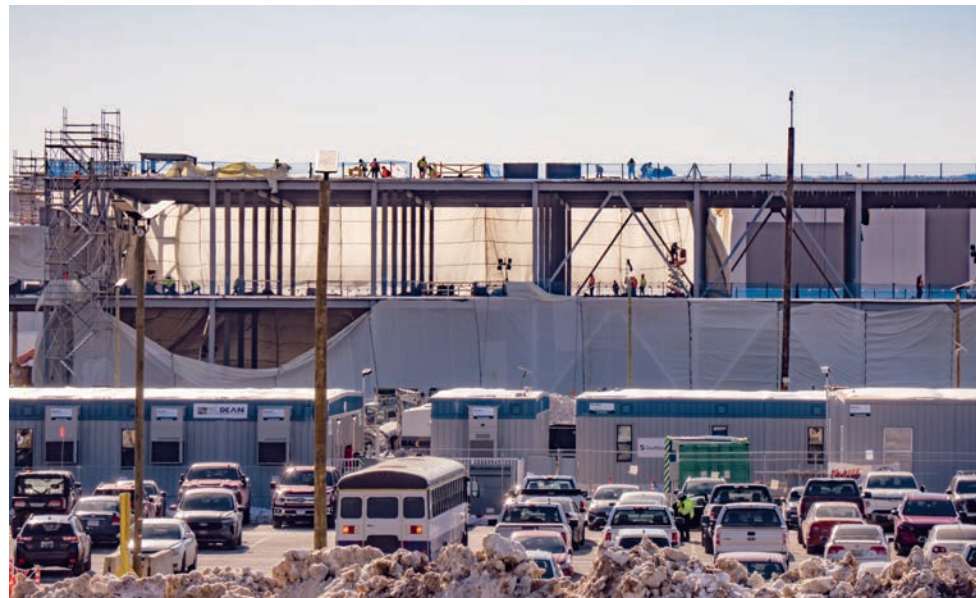
A new data center goes up in Frederick County, MD. (Dave Harp)
