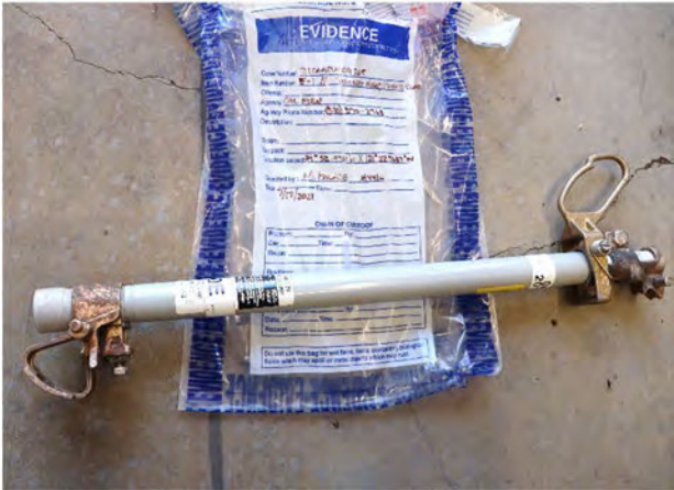
Figure 17: One of two fuses that operated
