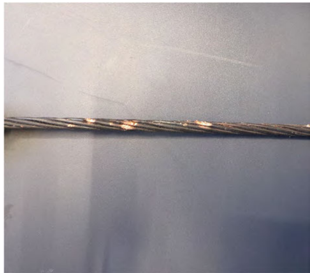
Figure 16: Signs of arcing from phase-to-phase contact on conductor
