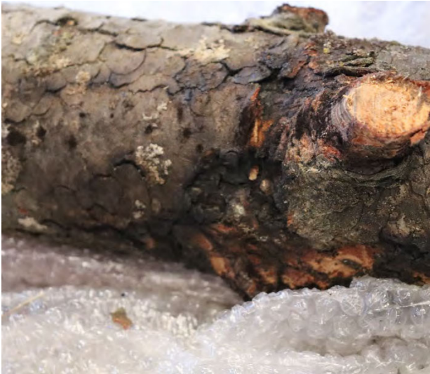
Figure 19: Subject Tree trunk where energized conductor contacted tree.
