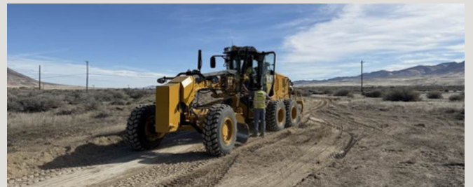
Above: Iron Horse, in partnership with Hunewill Construction Company, breaking ground at the Transload Terminal west of Winnemucca.
