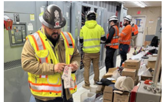
Target Construction and Ardent workers are pictured making final electrical connections at the WFH Main Electrical Switch.
