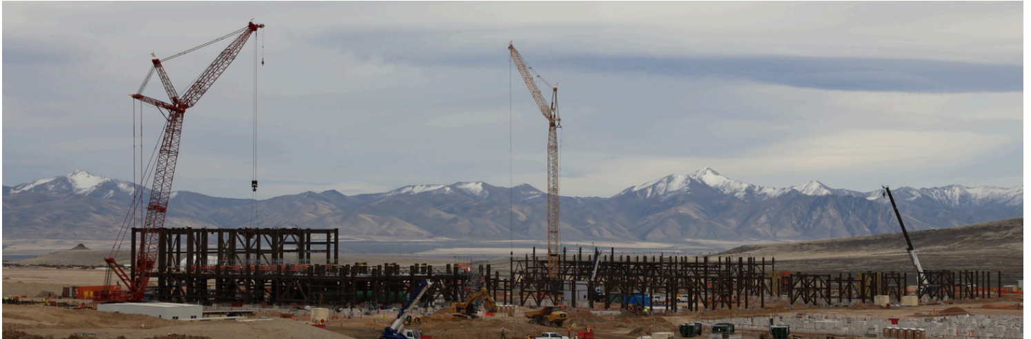
Structural steel advanced at the Filter Building, Magnesium Sulfate Building and Liquid Sulfur Tanks.
